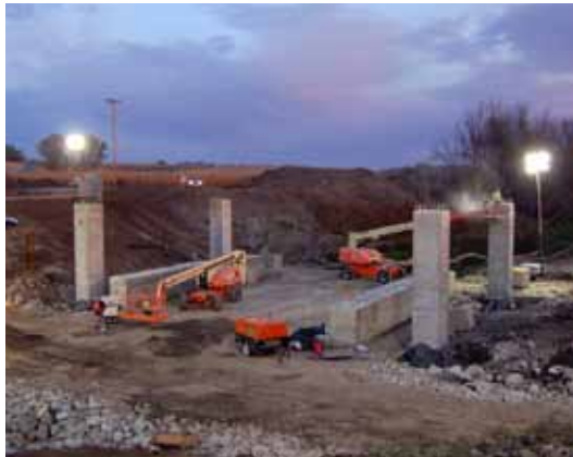
As part of a SHRP 2 demonstration of accelerated bridge construction techniques, Iowa DOT replaced a road bridge over Keg Creek in Pottawattamie County in October. The three-span, 210- by 47-ft structure was replaced with minimal disruption to traffic—it was closed for only two weeks. (Photo: Iowa DOT and HNTB)
