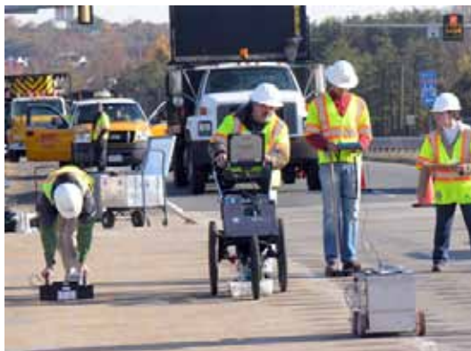
Nondestructive bridge testing techniques are among the research topics in the SHRP 2 renewal focus area.
