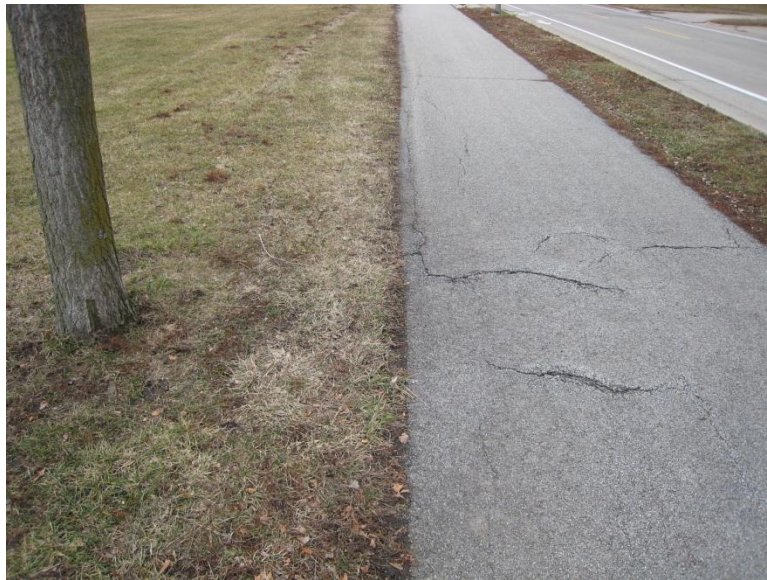
Figure D.15. Inadequate standoff and tree root infiltration.
