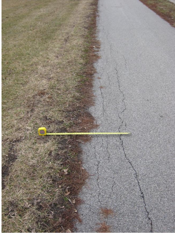
Figure D.14. Typical edge cracking on the east side of the trail.
