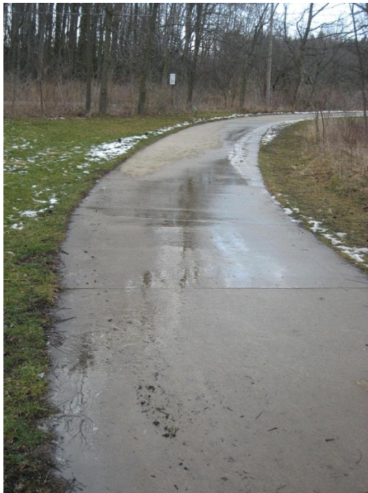
Figure D.4. Lack of trail drainage.
