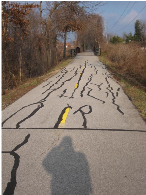
Figure D.35. Localized extreme longitudinal cracking.
