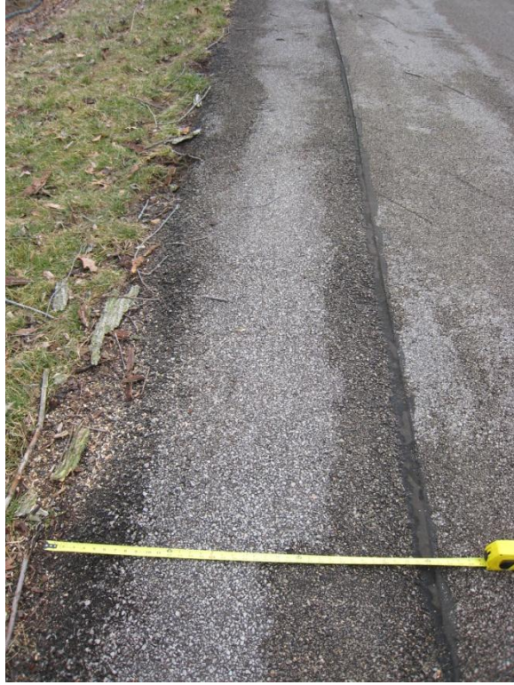
Figure D.34. Patch correcting edge cracking.
