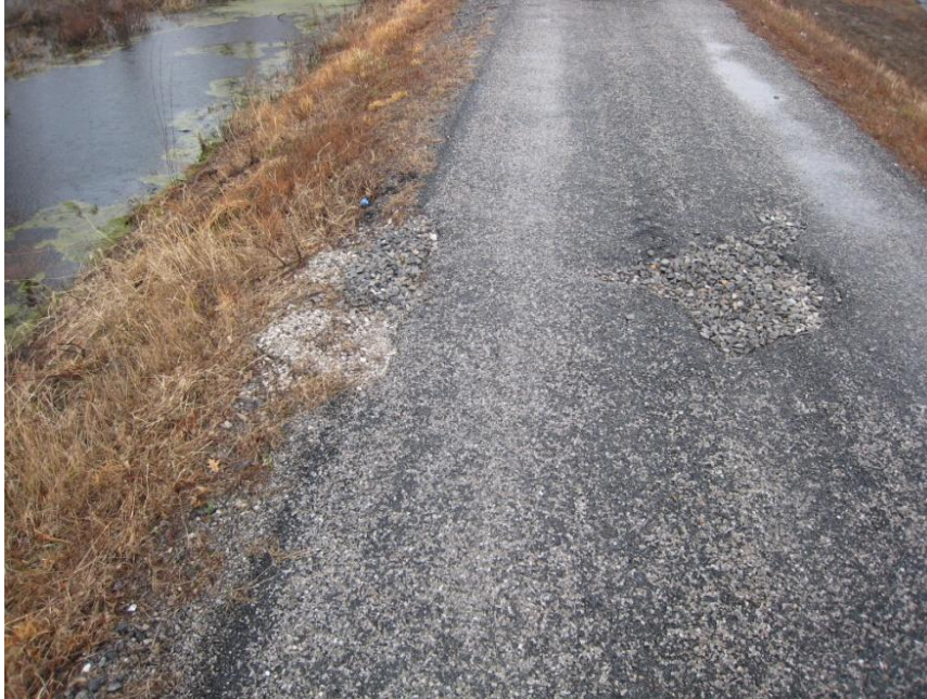
Figure D.29. Animal burrows causing surface collapses.
