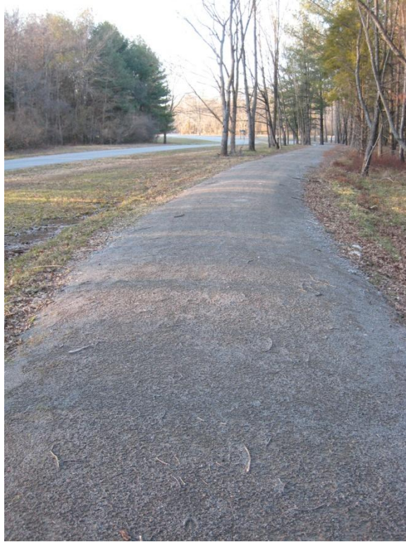
Figure D.22. Trail humping due to lack of shoulder material and no extension of aggregate base beyond aggregate surface.
