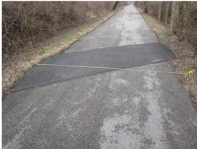
Figure D.33. Patch correcting tree root infiltration.
