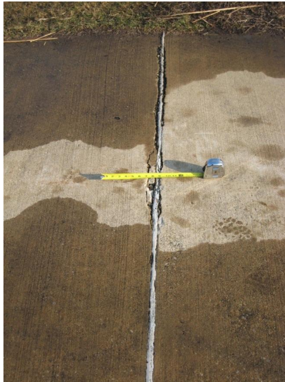
Figure D.6. Joint deterioration due to failing sealant.
