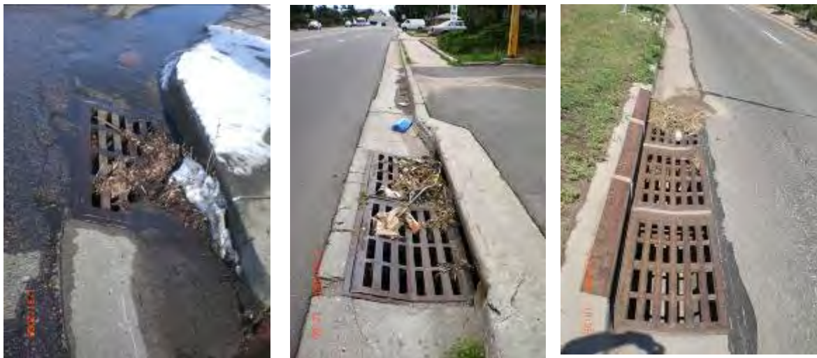
Figure 5.2 Decay of Debris Amount on Grates
