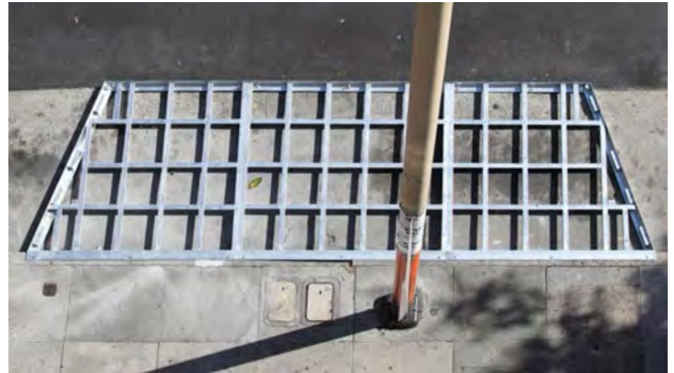
Figure 72. Installed steel sub-structure, "Peace Keeper" parklet, San Francisco, CA. Credit: Martha Traer
