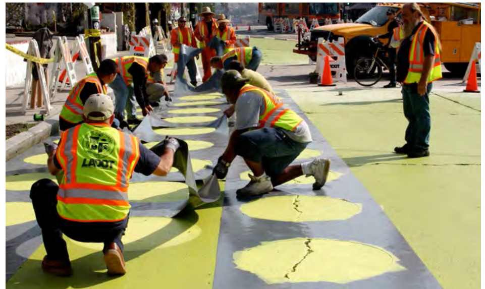
Figure 61. LADOT installation crews, Sunset Triangle Plaza, Los Angeles, CA. Credit: Margot Ocañas
