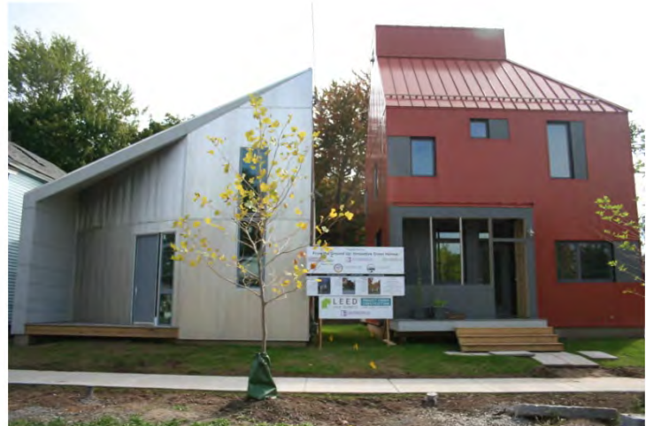
Figure 4. Single-family homes under construction in Syracuse, New York. These homes were built within an existing residential neighborhood not far from the city center. Photo credit: Syracuse Center of Excellence.
