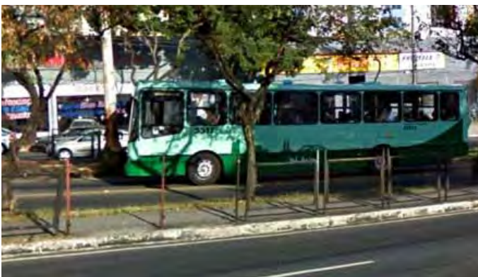
Guardrail along a Busway in Belo Horizonte, Brazil, damaged in order to allow crossing in mid-block. Photo by Carsten Wass.
