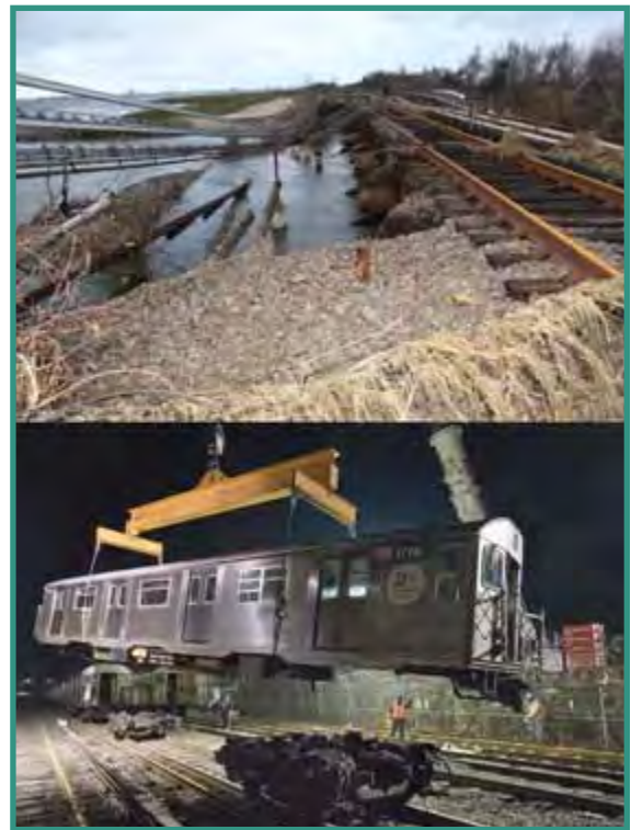
▲ Damaged and debris-strewn A train tracks, above; Transporting subway cars to the Rockaways, below. Photo Credits: MTA
