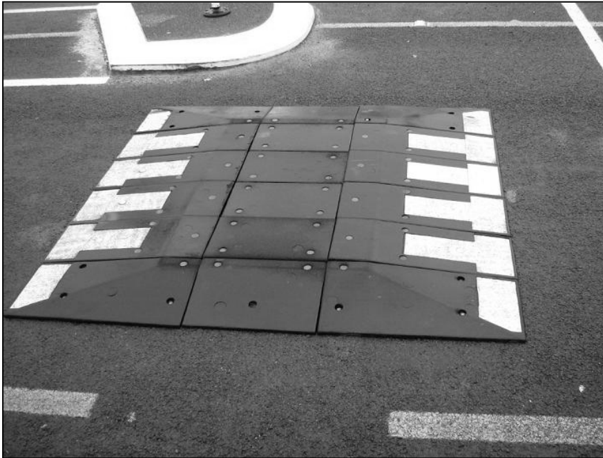
Figure 7.13 Photo of a 1.8m wide speed cushion installed on Pooks Road in Waitakere City (this 75mm high example is made of recycled rubber, which means it can be installed quickly and with minimum traffic management)
