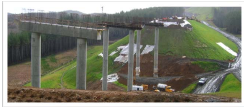
Figure 3.9: Construction of a bridge on the U.S. 20 Pioneer Mountain to Eddyville realignment project. The white tarps on the hillside cover the superficial slope failures, which have resulted in substantial cost and time delays to the project.
