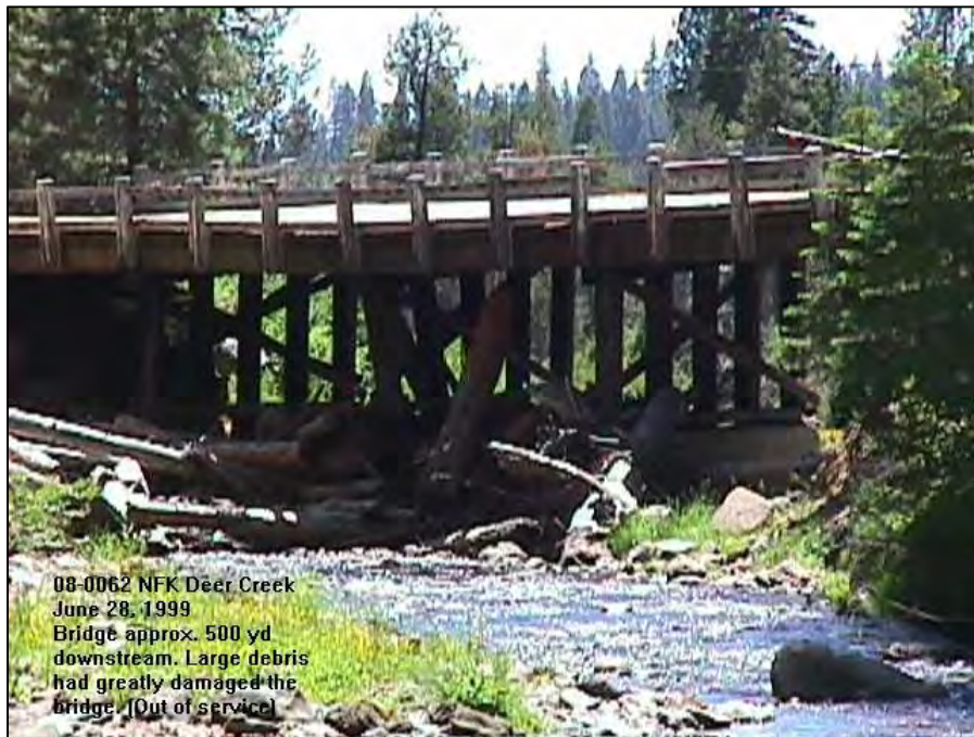
Figure 5.7 Structurally Deficient – Low Substructures Condition Rating & Low Waterway Adequacy
