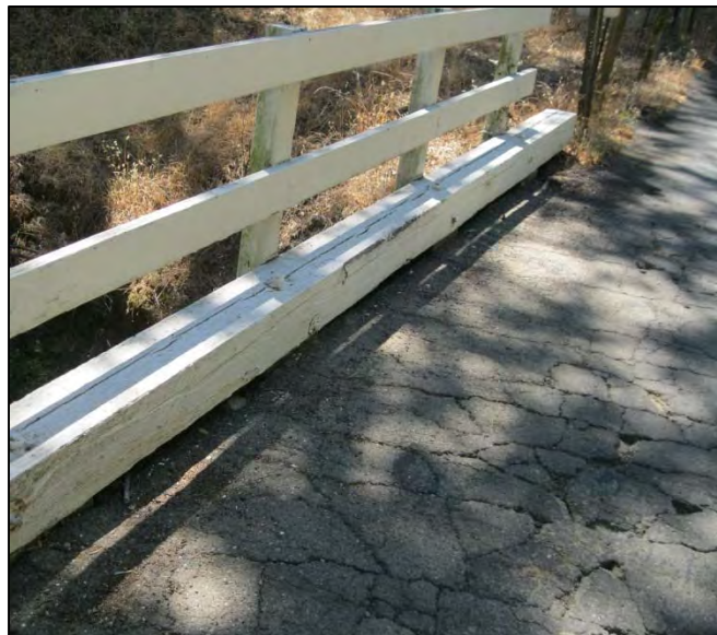
Figure 5.11 Bridge Deck Requiring Replacement
