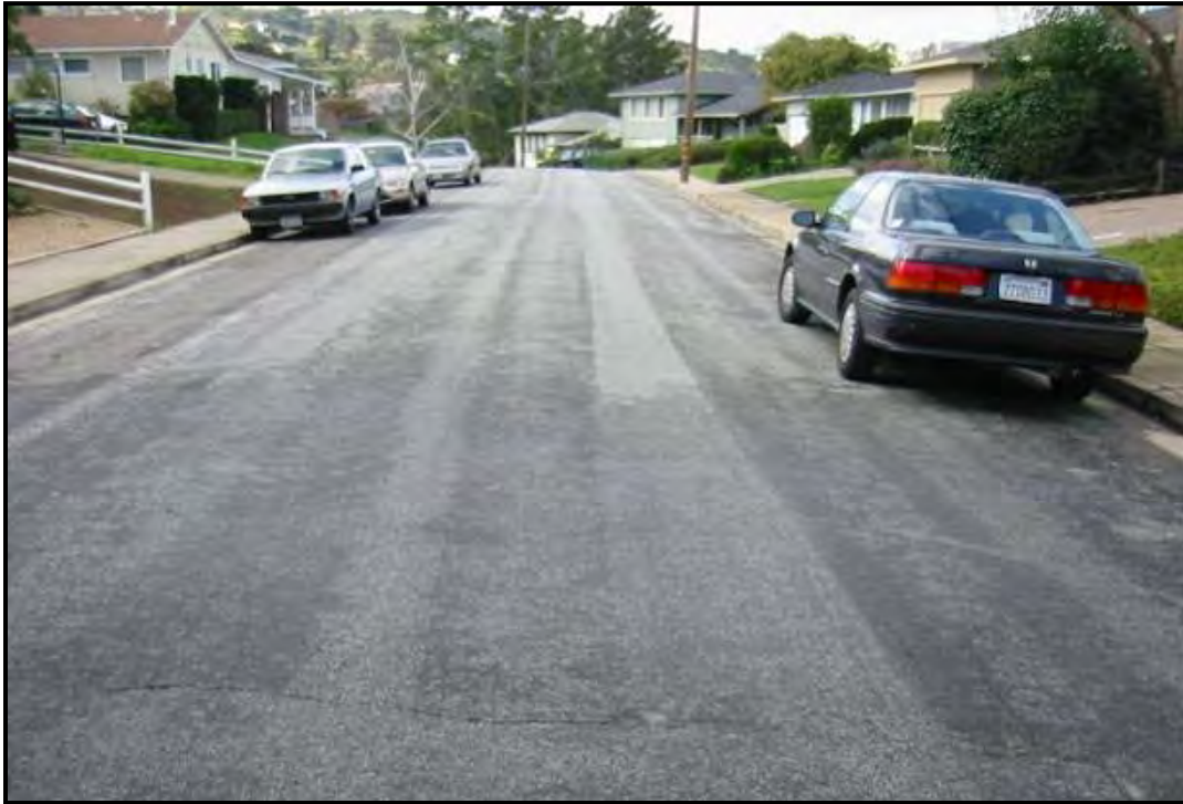
Figure 2.6 Example of Local Street with PCI = 66
