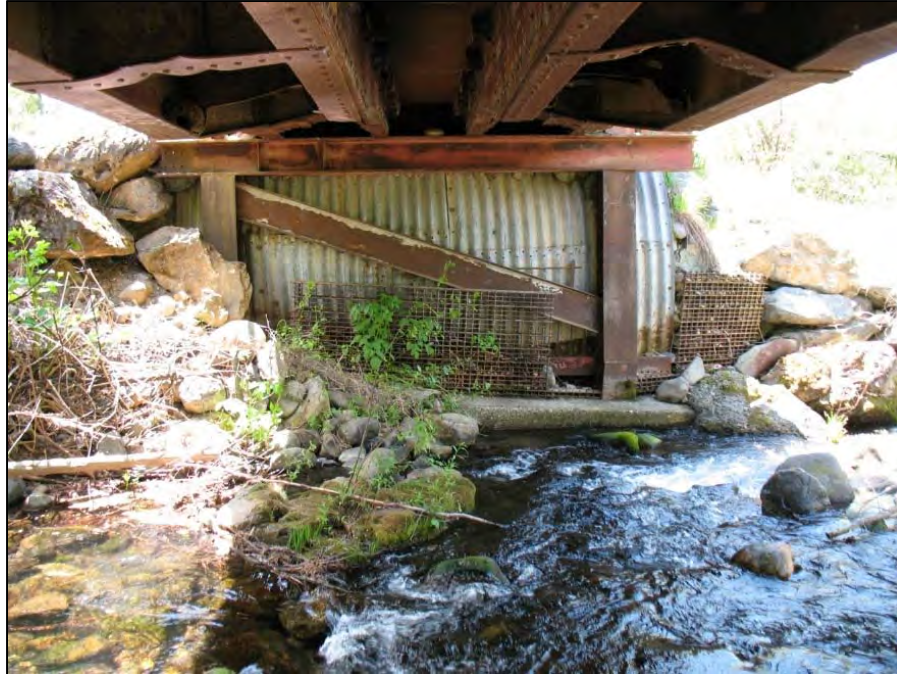
Figure 5.6 Structurally Deficient – Low Superstructure & Substructures Condition Rating
