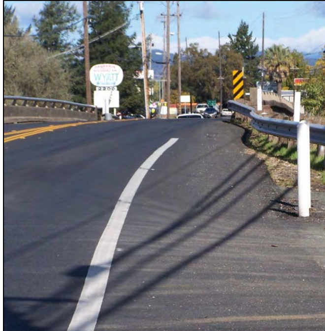
Figure 5.8 Functionally Obsolete – Low Approach Roadway Alignment Appraisal Rating
