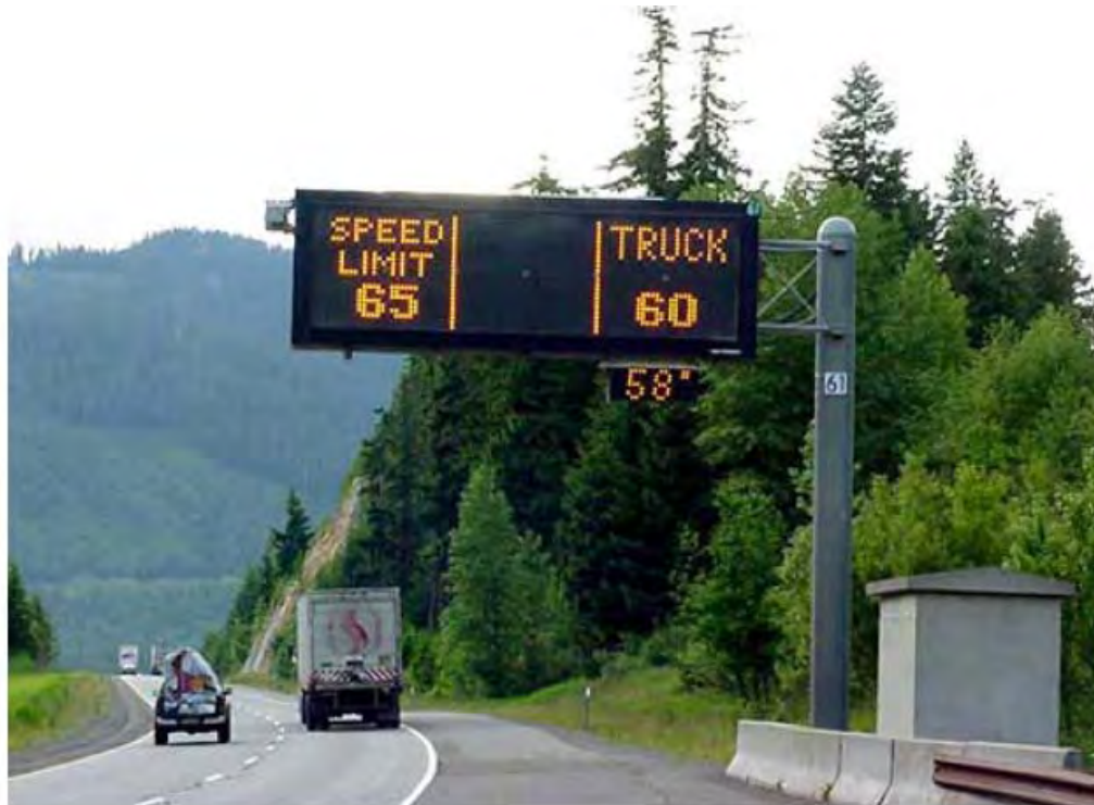
Figure 2.4: Variable Speed Limit Sign used on I-90 on Snoqualmie Pass in Washington. (Source: Washington State Department of Transportation)
