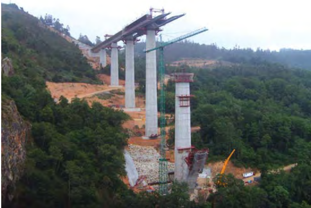
Construction of high-speed rail lines in other countries has created thousands of jobs. Here, construction is underway on a bridge as part of Spain's efforts to extend its high-speed rail network. Credit: Xosema, used under Creative Commons license
