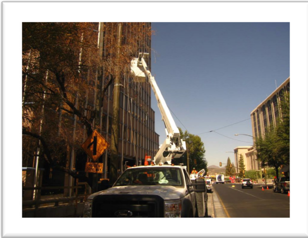
Figure 3-4 Typical OCS Installation (Tucson, AZ)
