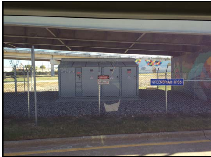
Dallas Sample Streetcar Traction Power Substation Units (HDR 2013)
