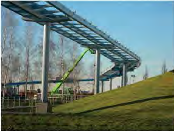
Elevated carriageway is light weight and easy to construct using off-site prefabricated elements.
