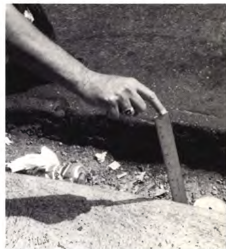
Cracks and potholes are estimated to cost each car driver $100 a year in auto repairs.
