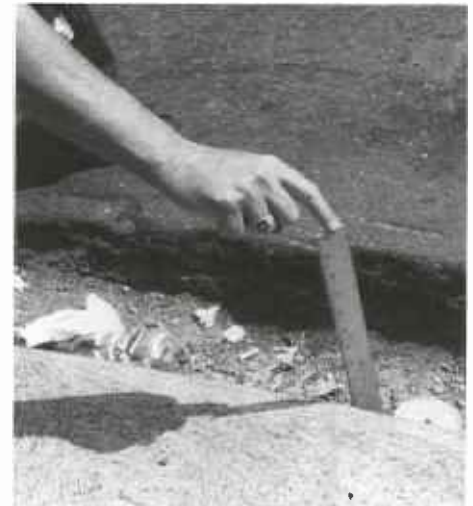
Cracks and potholes are estimated to cost each car driver $100 a year in auto repairs.
