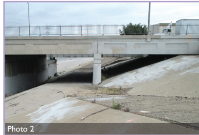
Photo 2 Location of the existing maintenance access road North of Downey Road, looking South.
