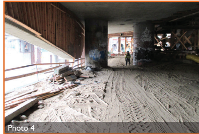
Top of bank area at historic Riverside Drive bridge footing. Taken during Riverside Drive Bridge replacement, looking South.
