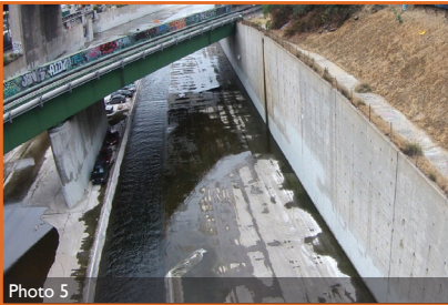
Location of the existing Union Pacific railroad crossing North of SR-110, looking South to the confluence with Arroyo Seco.
