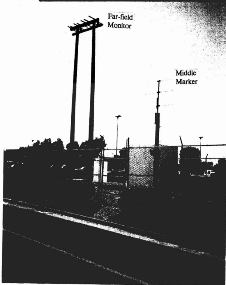
Figure 3-1b. Runway 24R Middle Marker Installation with Center Far-field Monitor Antenna.
