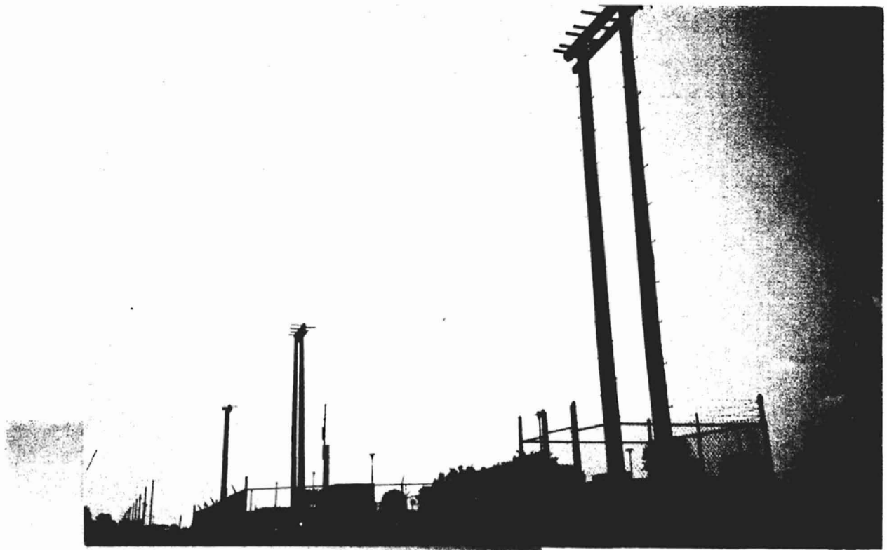
Figure 3-1a. Runway 24R Localizer Far-field Monitor Antennas and Middle Marker.
