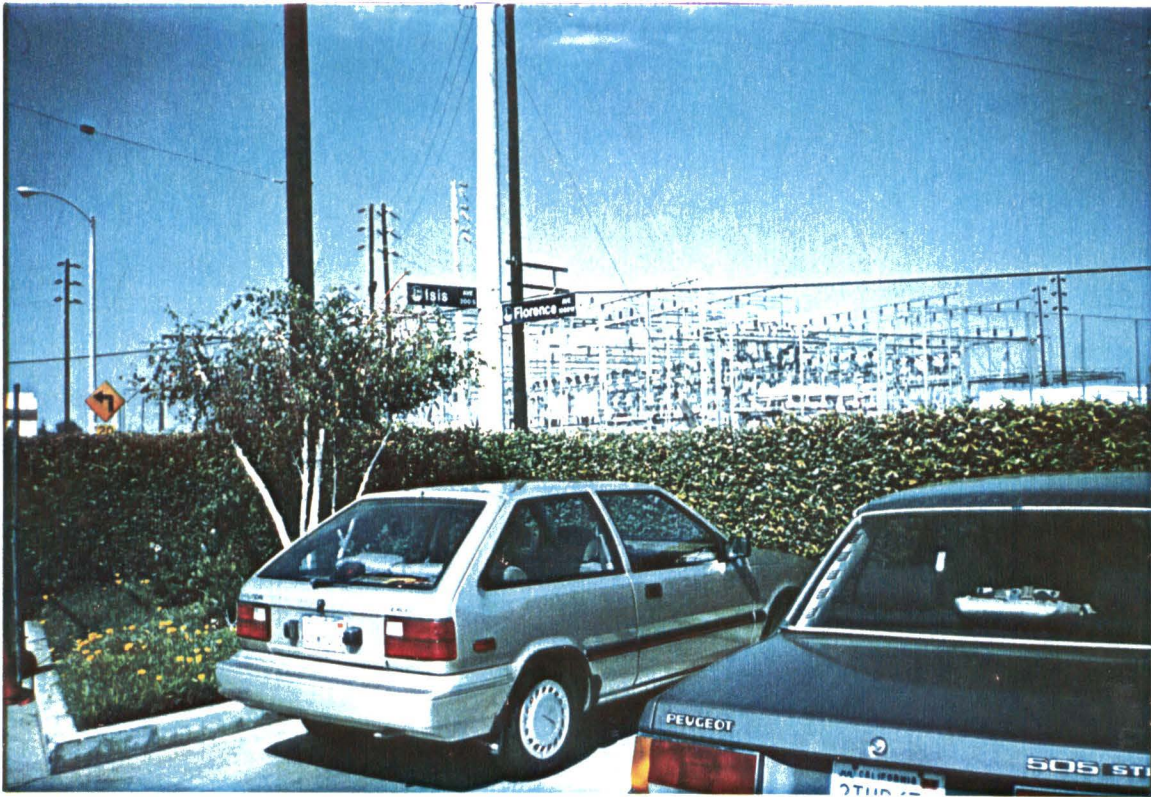
FIGURE 1.5 LAX TO MARINA FREEWAY (STATION 1 TO 2) FLORENCE AVENUE & ISIS AVENUE - DWP SUBSTATION
