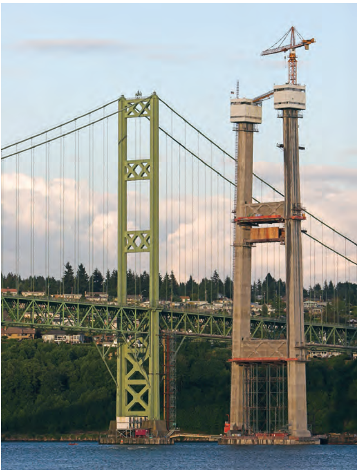
Old and new: Nearly 60 years' worth of bridge design advances—many supported by NCHRP research—are evidenced in the construction of the twin spans of the Tacoma Narrows bridge in Washington state.
