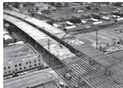
Highways rise up in Florida: The Interstate construction boom in the late 1950s and early 1960s drove the need for cooperative research efforts. (Image courtesy of Florida Department of State)
