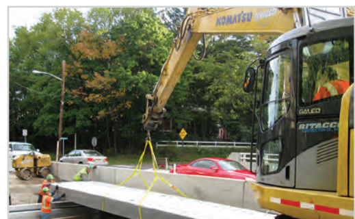
A hybrid-composite beam is lowered into place as a New Jersey bridge takes shape. The NCHRP IDEA Program (Project 20-30) helped put the innovative new bridge beam concept into practice.
