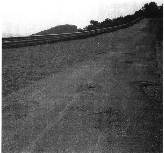
Figure 15 Service lane pavement damage from vehicle removal activities.
