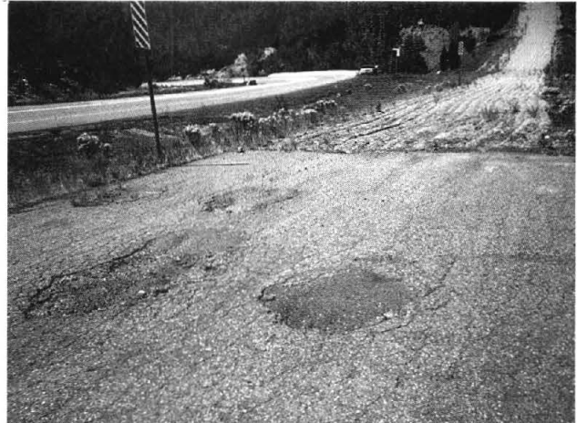
Figure 14 Apron pavement damage probably caused by truck retrieval.
