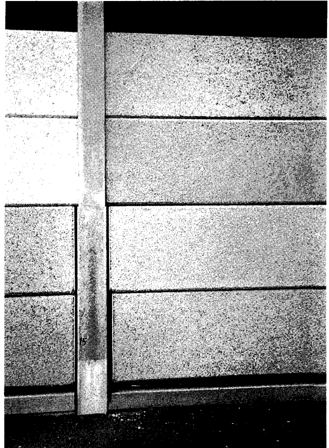
FIGURE 7 Ontario panel hinged to release floodwaters trapped on road side of barrier.
