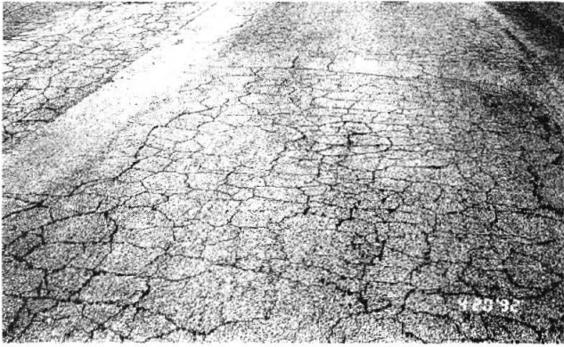
Figure 8 An old asphalt pavement that has surface cracks but has maintained good structural integrity is suitable for hot in-place recycling.
