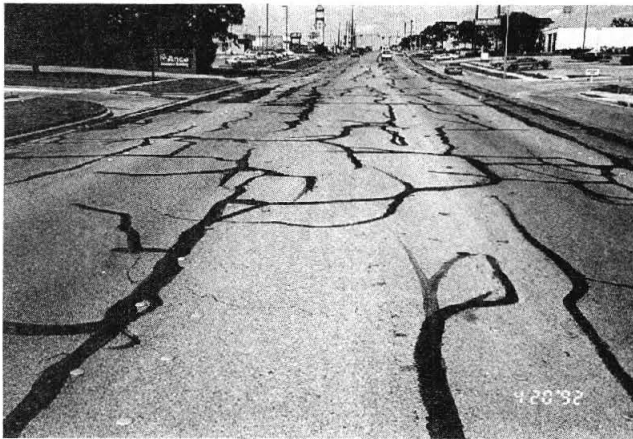
Figure 9 Ride quality of this pavement may be restored by HIPR but removal of excessive crack sealer may be required in some areas.
