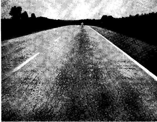
FIGURE 33 A well-defined crack pattern associated with the development of ASR in highway pavement. (Source: SHRP)
