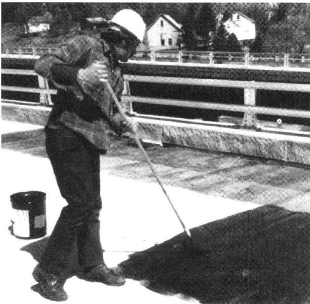
FIGURE 15 Application of a proprietary primer using a roller. (Courtesy of Vermont Agency of Transportation)
