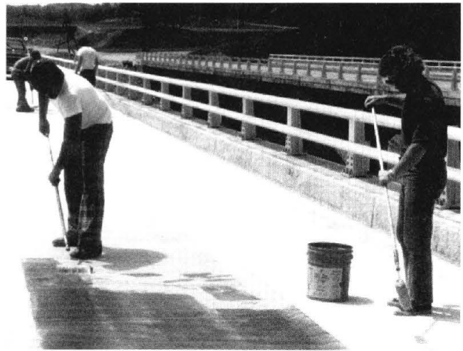
FIGURE 16 Applying adhesive to the deck and an EPDM rubber sheet. (Courtesy of Vermont Agency of Transportation)
