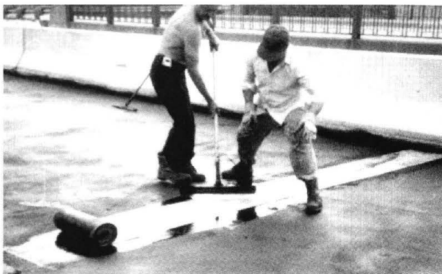
FIGURE 12 Use of a strip of preformed sheet embedded in liquid membrane at a construction joint in the deck.
