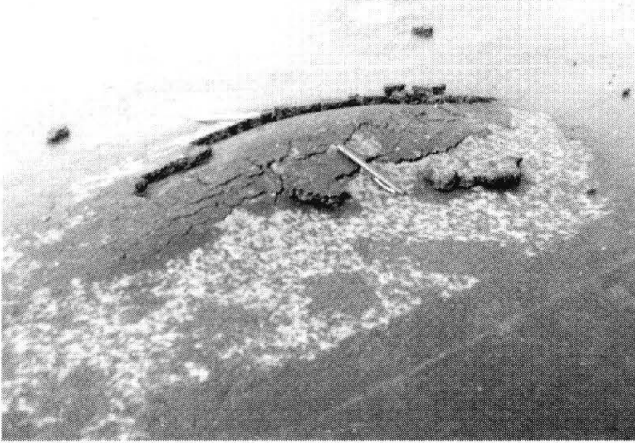
FIGURE 23 Blisters in membrane and base course. (Courtesy of Vermont Agency of Transportation)
