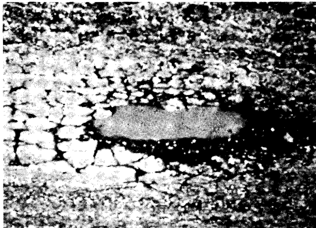
FIGURE A-3 Pothole (20).
