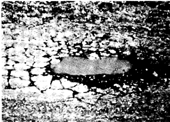
FIGURE A-3 Pothole (20).
