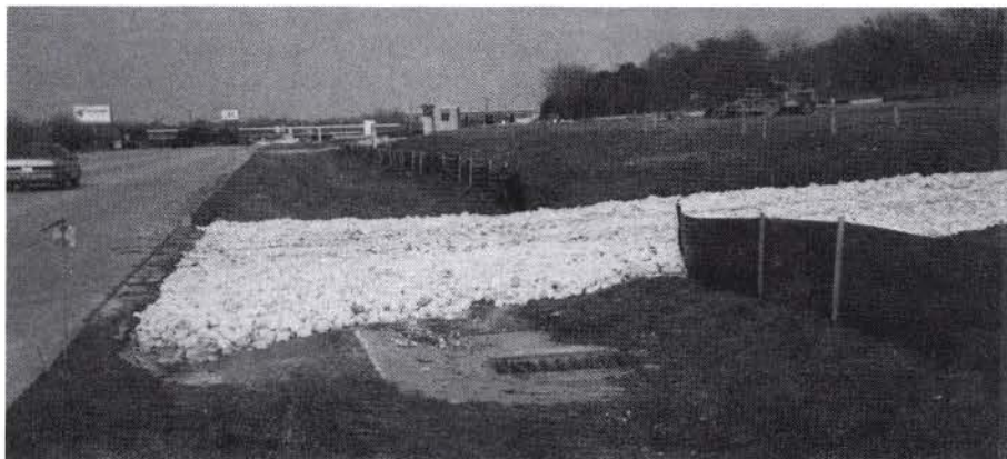
FIGURE 13 Good use of BMPs.
