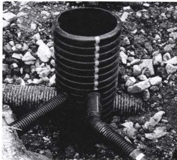
FIGURE 18 Low maintenance, dual pipe edgedrain with ditch line collector used in Kentucky: (a) loop edgedrain with ditch line collector; (b) inspection port (Fleckenstein and Allen 1999).
