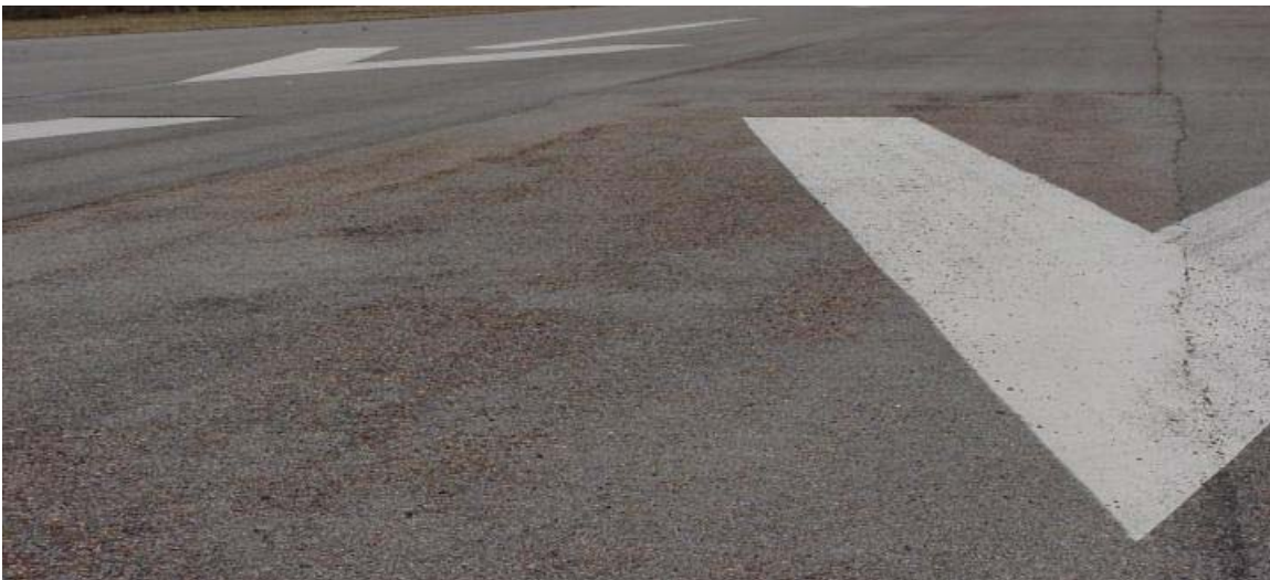
Figure 5-15. Weathering and raveling caused due to loss of pavement binder
