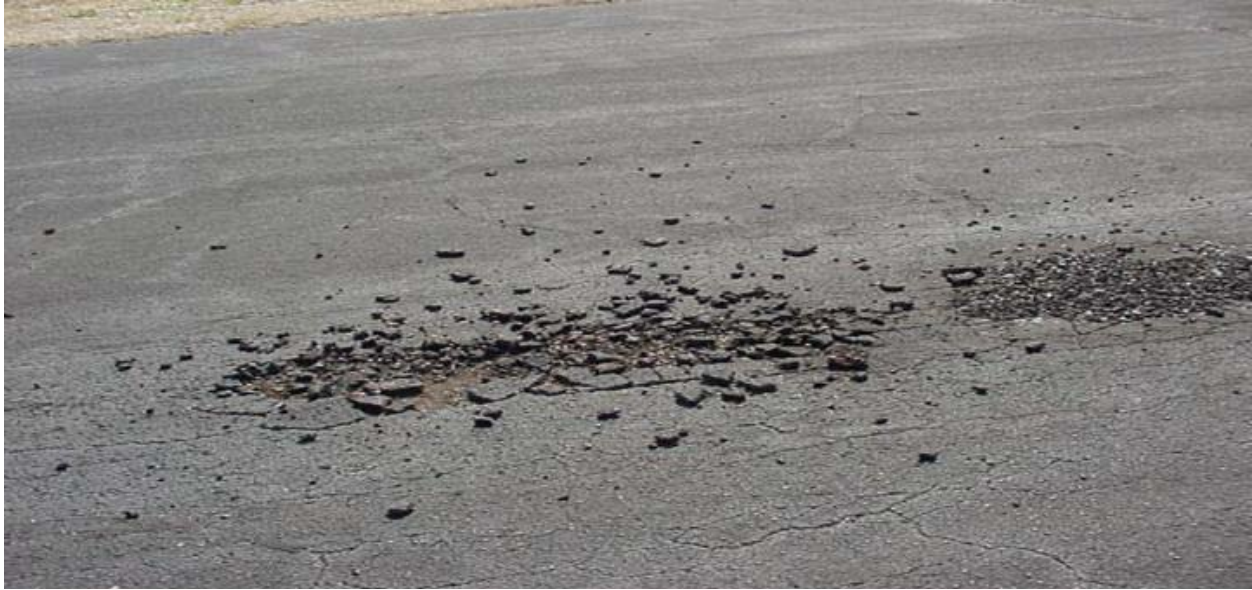
Figure 5-11. Severe alligator cracking that caused potholes
