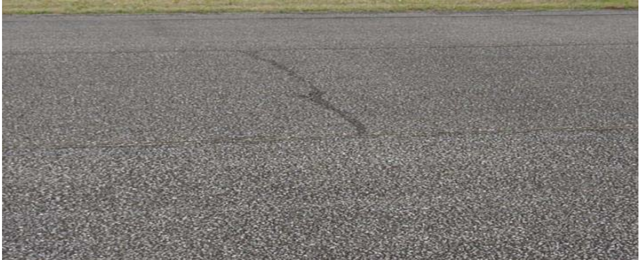
Figure 5-17. Longitudinal cracks connected by transverse cracks
