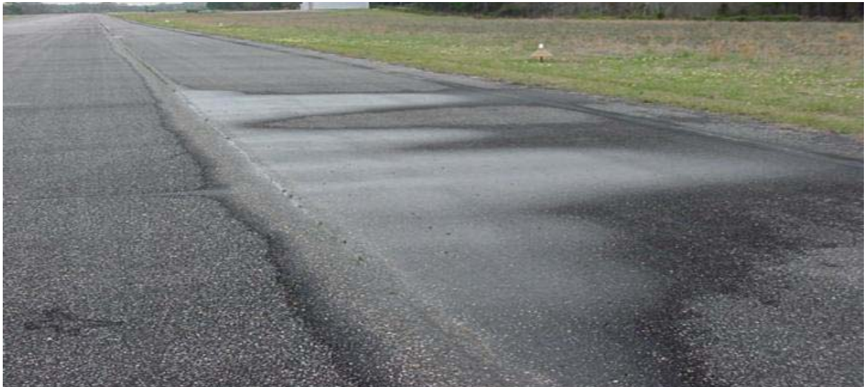
Figure 5-18. Water seeping out through longitudinal crack due to load application
