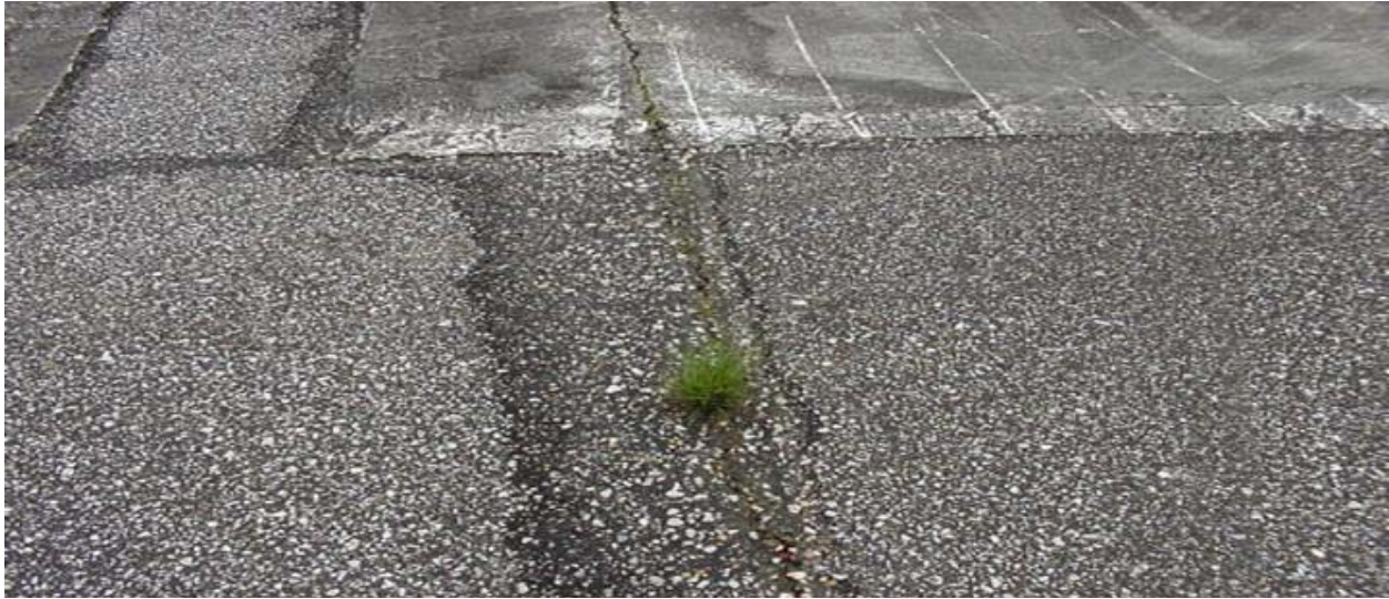
Figure 5-16. Weathered pavement with grass sprouting along cracks
