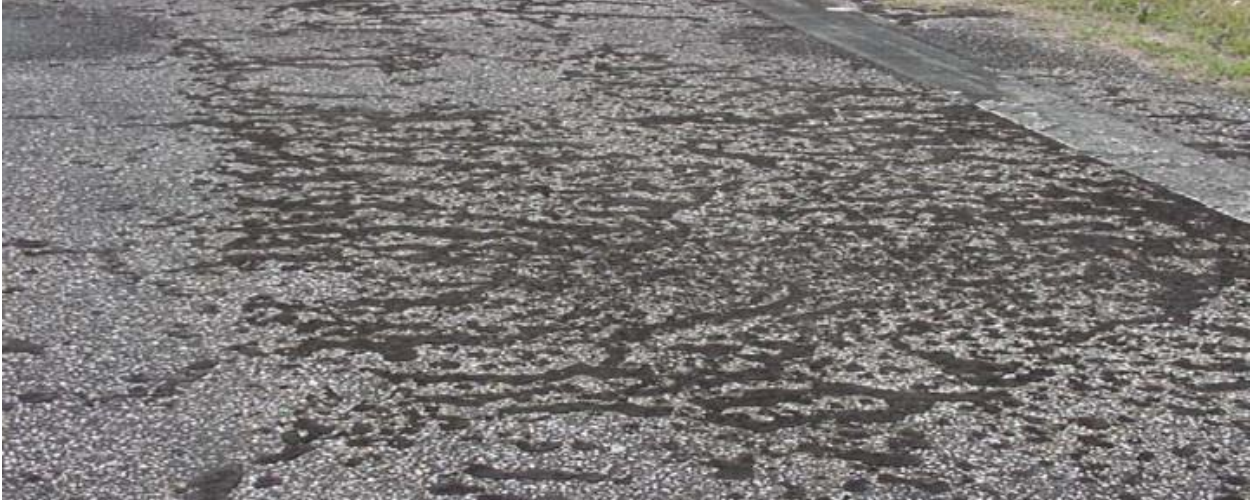
Figure 5-19. Mild asphalt bleeding along pavement strip
