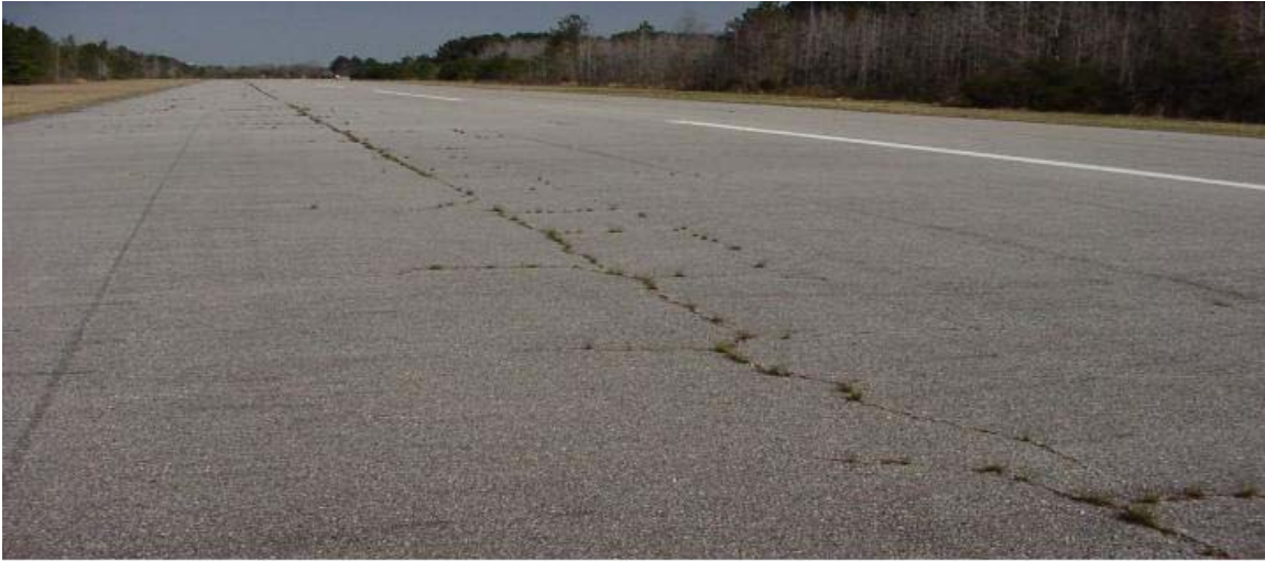
Figure 5-14. Grass sprouting along cracks
