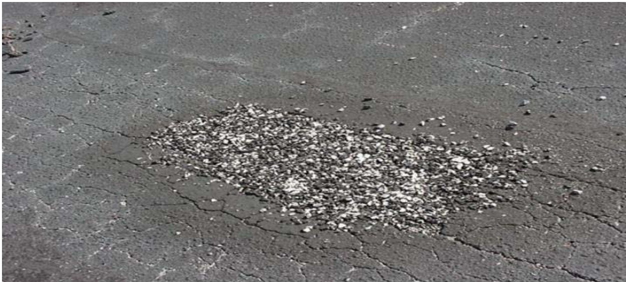
Figure 5-12. Poorly patched potholes
