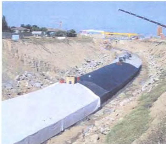
Applying the waterproofing layer to the external roof of the cut and cover tunnel.
