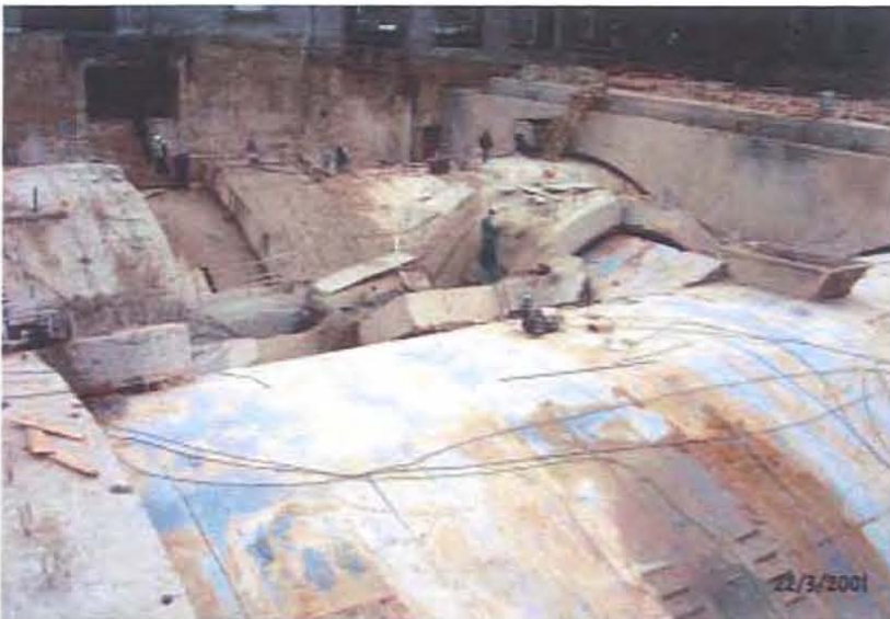
Transverse cuts for the introduction of steel framework over RENFE line tunnels.
