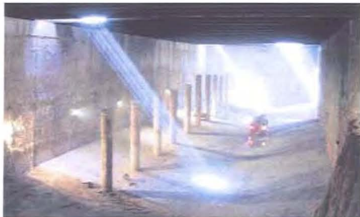
Beamed roof and invert slab with mezzanine support pillars at Alcorcón 3 station.
