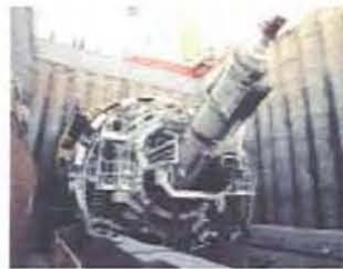
View of the screw conveyor
