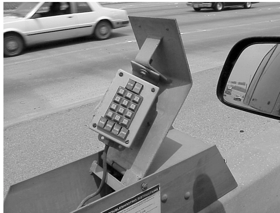
Figure 3-11. EA BarrierGate Controls.
