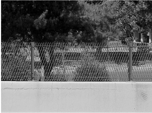
Figure 8-2. Chain Link Glare Screen.
