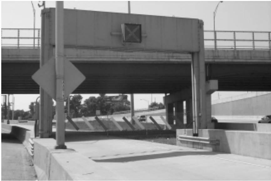
Figure 3-14. Fiber-Optic Sign on Barrier Structure (Enhanced Digitally to Show Indication).
