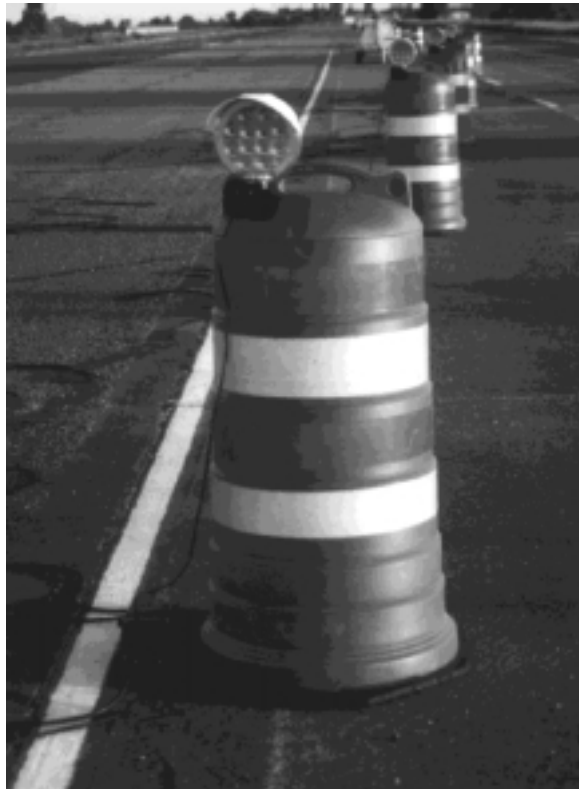
Figure 2. Individual Flashing Warning Light Connection.
