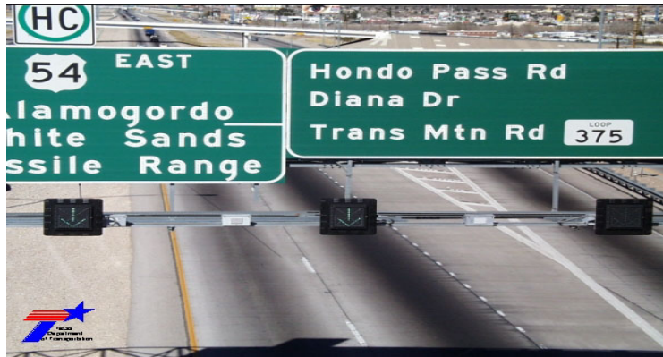
Figure 6. Overhead Lane Control Signal in El Paso ( 11 )
