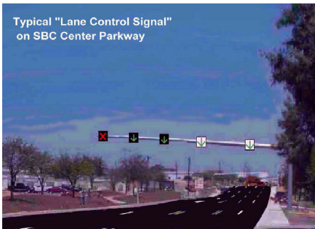
Figure 18. SBC Parkway Lane Control Signal
