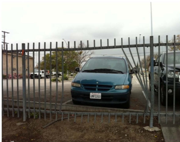
Figure 5 -12. Gates at Vermont Station are damaged and not maintained.
