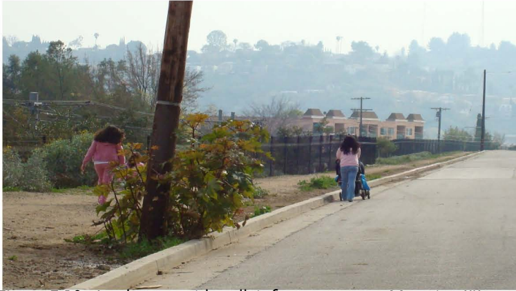
Figure 7-10. Inadequate sidewalk infrastructure on Marmion Way.
