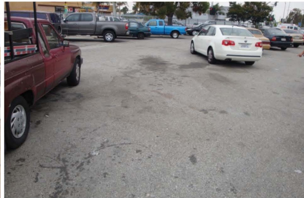
Figure 5-15. Striping is faded, partly from oil leaks.
