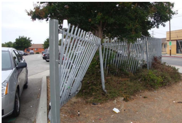
Figure 5-14. Fences surrounding the Northwest Lot are broken causing a safety hazard.
