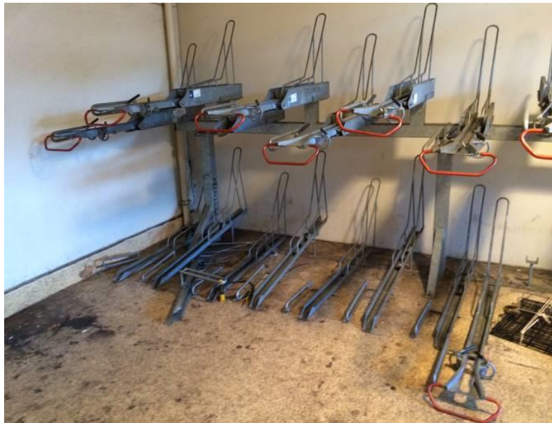
Photo 79: Poorly Maintained Bicycle Storage Room
