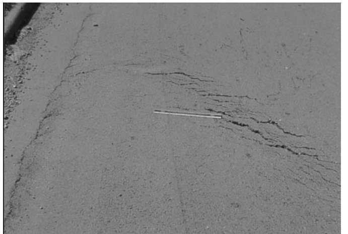
FIG. X1.48 Medium-Severity Slippage Cracking
