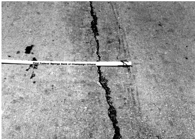
FIG. X2.23 Medium-Severity Linear Cracking
