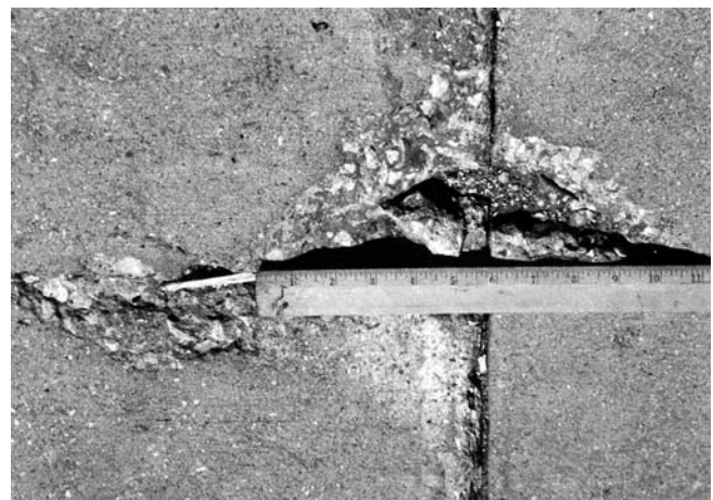
FIG. X2.46 Medium-Severity Spalling, Corner
