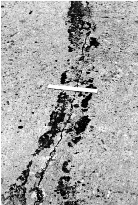
FIG. X2.22 Low-Severity Linear Cracking
