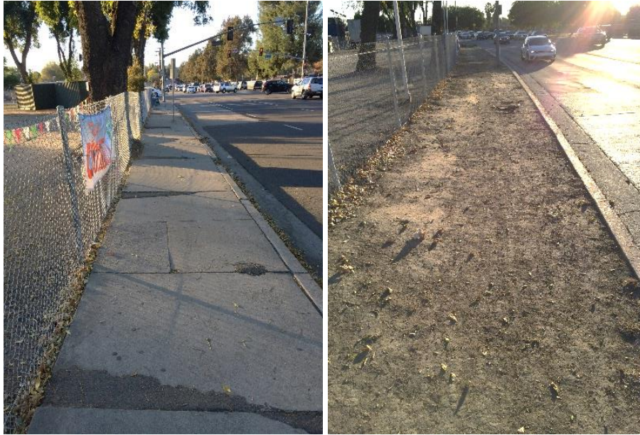
Photo 190: Buckled Sidewalk near Station (L); Where Sidewalk Ends on Victory Blvd. east of Winnetka Ave. (R)
