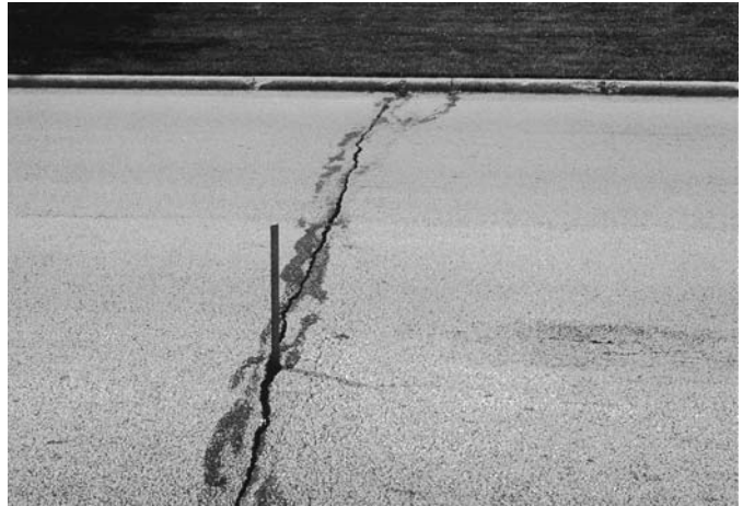
FIG. X1.29 Medium-Severity Longitudinal and Transverse Cracking
