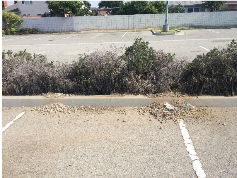
Photo 244: Poorly Maintained Landscaping and Litter in Parking Lot
