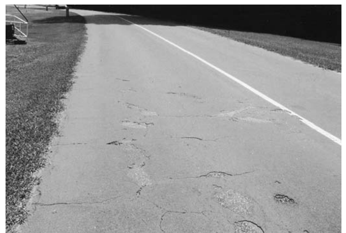
FIG. X1.53 High-Severity Weathering and Raveling
