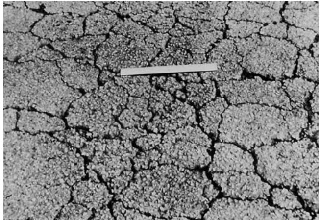
FIG. X1.3 High-Severity Alligator Cracking
