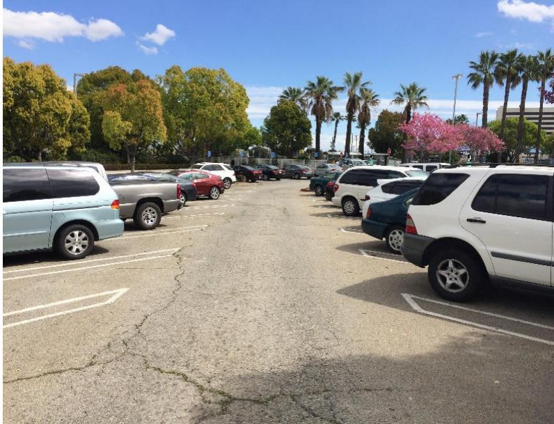
Photo 14: Cracks in the Pavement
