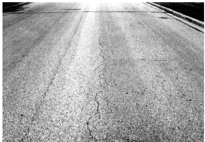
FIG. X1.1 Low-Severity Alligator Cracking
