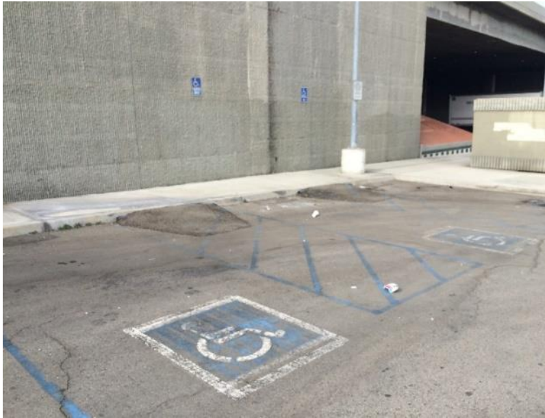
Photo 221: Non-Compliant ADA Ramps
