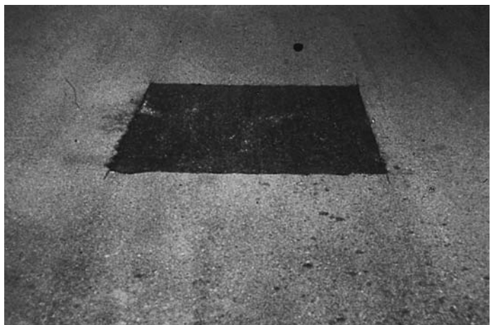
FIG. X1.31 Low-Severity Patching and Utility Cut Patching
