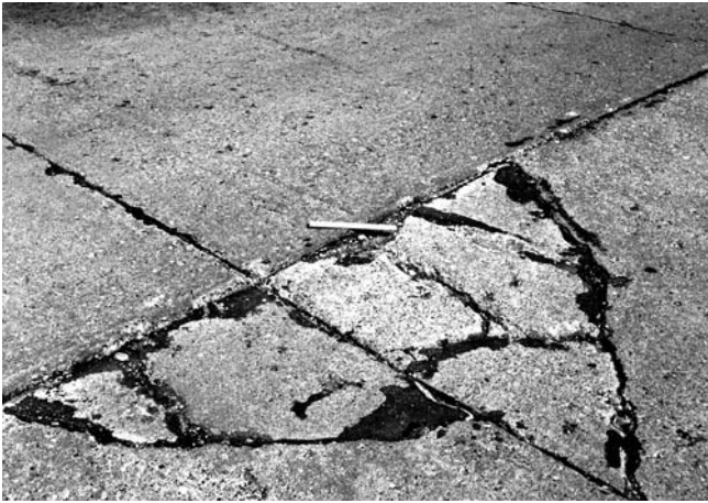
FIG. X2.6 High-Severity Corner Break
