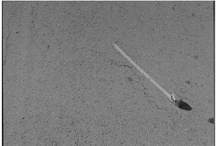
FIG. X1.47 Low-Severity Slippage Cracking
