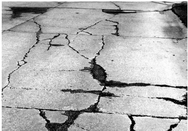
FIG. X2.9 High-Severity Divided Slab
