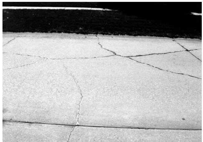
FIG. X2.8 Medium-Severity Divided Slab
