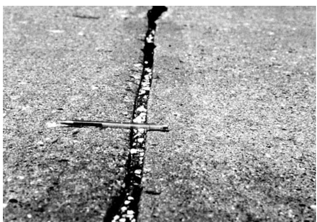
FIG. X2.18 High-Severity Joint Seal Damage
