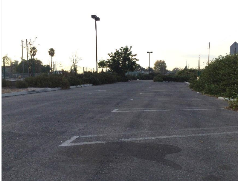
Photo 6: Faded Parking Space Striping
