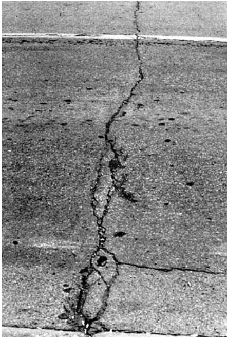
FIG. X1.23 Medium-Severity Joint Reflection Cracking
