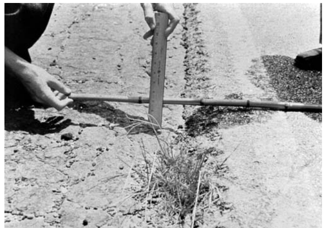
FIG. X1.26 Medium-Severity Lane/Shoulder Drop-Off
