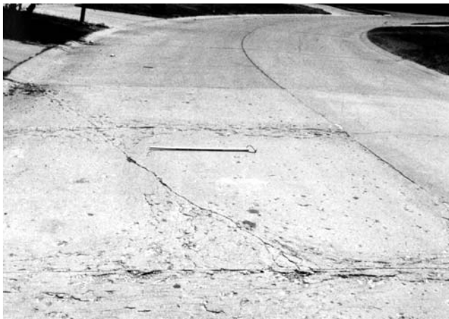
FIG. X2.12 High-Severity Durability Cracking
