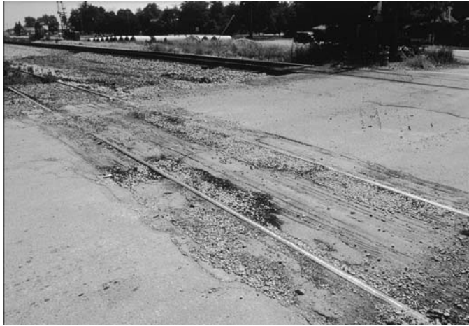
FIG. X1.40 High-Severity Railroad Crossing
