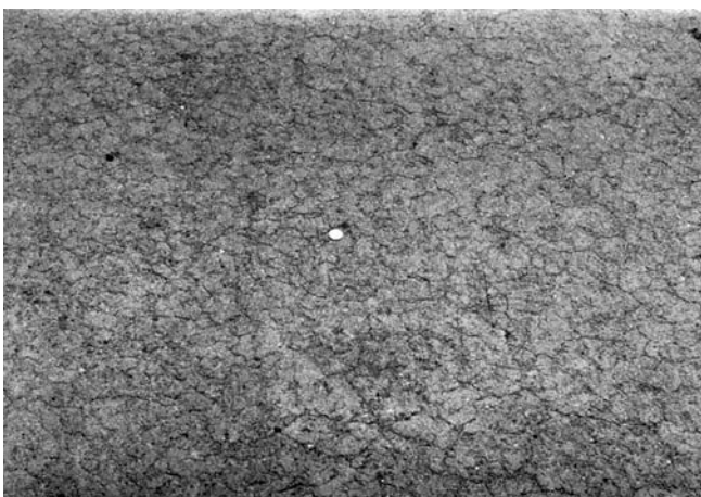
FIG. X2.41 Low-Severity Scaling, Map Cracking, and Cracking
