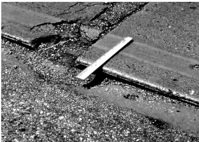
FIG. X2.19 Low-Severity Lane/Shoulder Drop-Off
