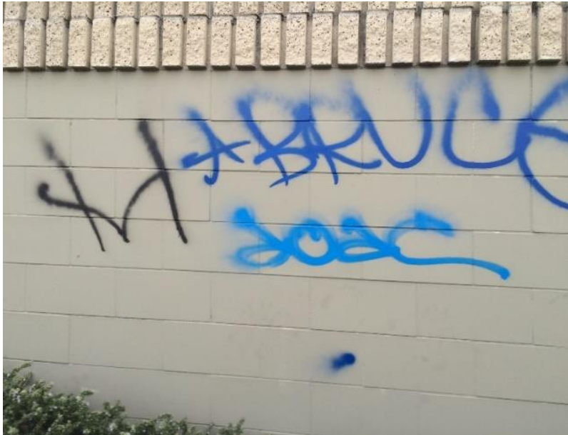
Photo 227: Graffiti on side of Utility Building
