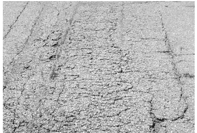
FIG. X1.52 Medium-Severity Weathering and Raveling
