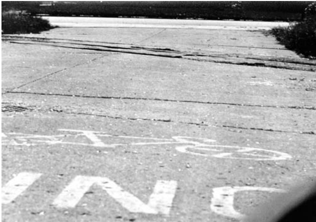
FIG. X2.39 Medium-Severity Railroad Crossing
