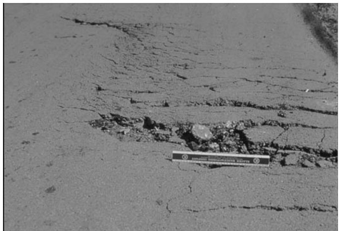
FIG. X1.49 High-Severity Slippage Cracking
