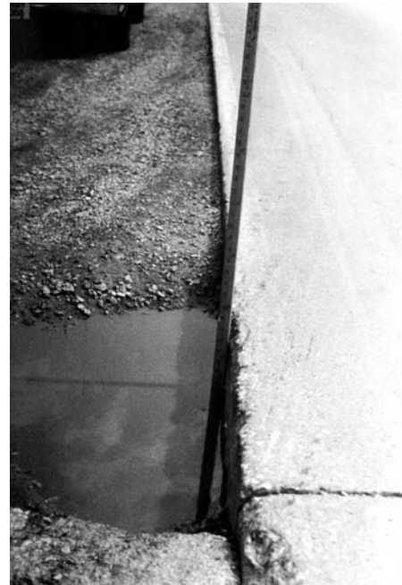
FIG. X2.21 High-Severity Lane/Shoulder Drop-Off
