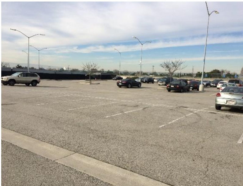
Photo 228: Cracked Pavement in Lot
