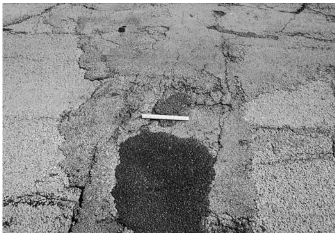
FIG. X1.33 High-Severity Patching and Utility Cut Patching
