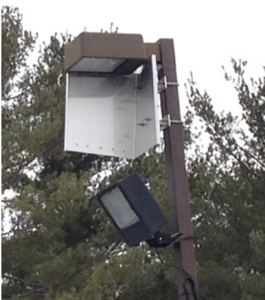
Figure 5. A floodlight had to be added to supplement the light absorbed by the shield mounted on the parking lot luminaire.
