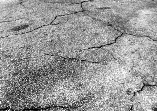
FIG. X1.9 High-Severity Block Cracking
