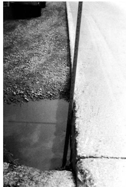
FIG. X2.21 High-Severity Lane/Shoulder Drop-Off
