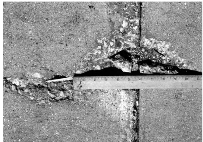
FIG. X2.46 Medium-Severity Spalling, Corner
