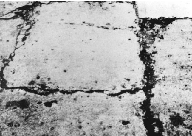
FIG. X2.27 High-Severity Patching, Large and Utility Cuts
