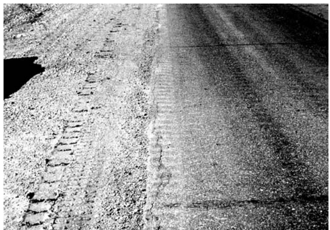
FIG. X1.22 Low-Severity Joint Reflection Cracking
