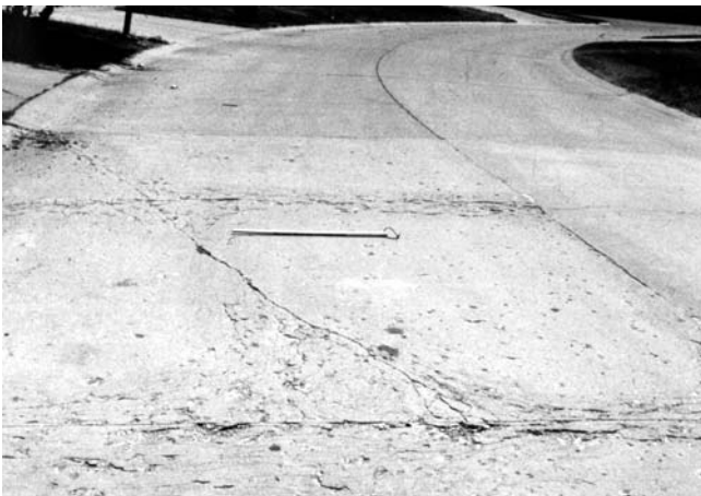
FIG. X2.12 High-Severity Durability Cracking
