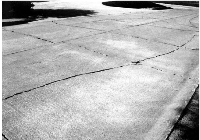
FIG. X2.7 Low-Severity Divided Slab
