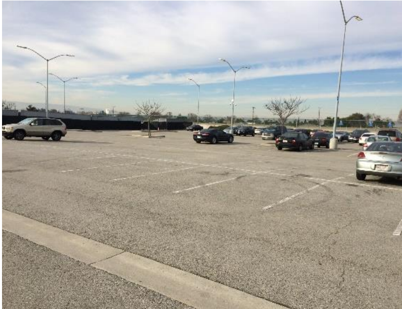
Photo 228: Cracked Pavement in Lot
