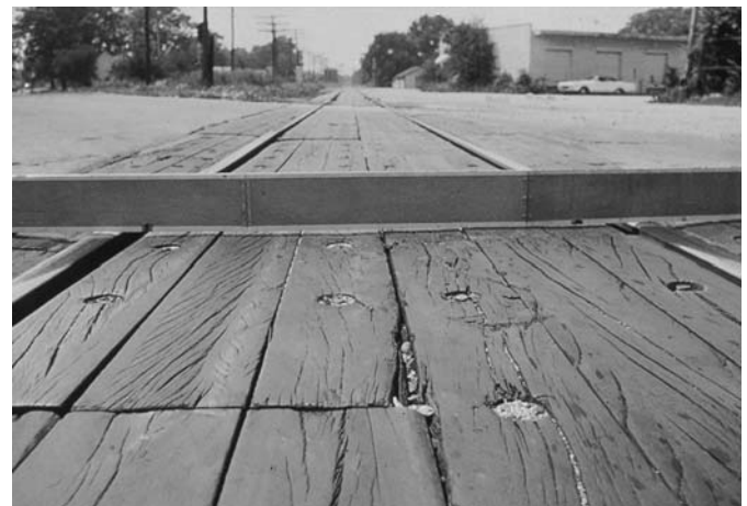
FIG. X1.38 Low-Severity Railroad Crossing
