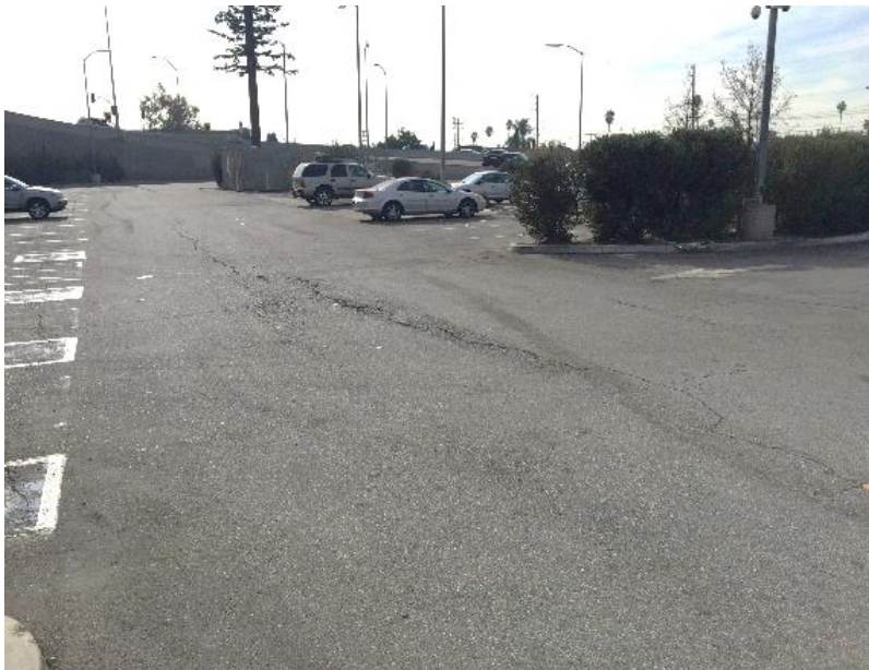
Photo 220: Pavement Cracking in Lot
