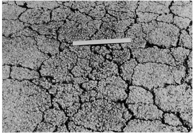
FIG. X1.3 High-Severity Alligator Cracking
