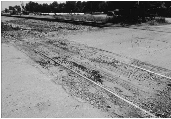
FIG. X1.40 High-Severity Railroad Crossing
