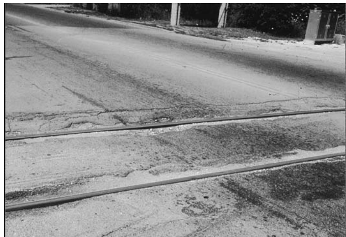
FIG. X1.39 Medium-Severity Railroad Crossing
