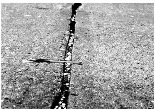
FIG. X2.18 High-Severity Joint Seal Damage
