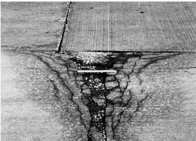
FIG. X2.11 Medium-Severity Durability Cracking
