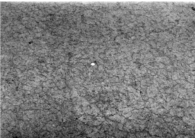
FIG. X2.41 Low-Severity Scaling, Map Cracking, and Cracking
