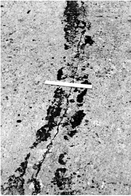
FIG. X2.22 Low-Severity Linear Cracking
