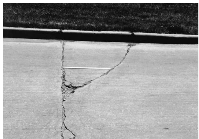
FIG. X2.5 Medium-Severity Corner Break
