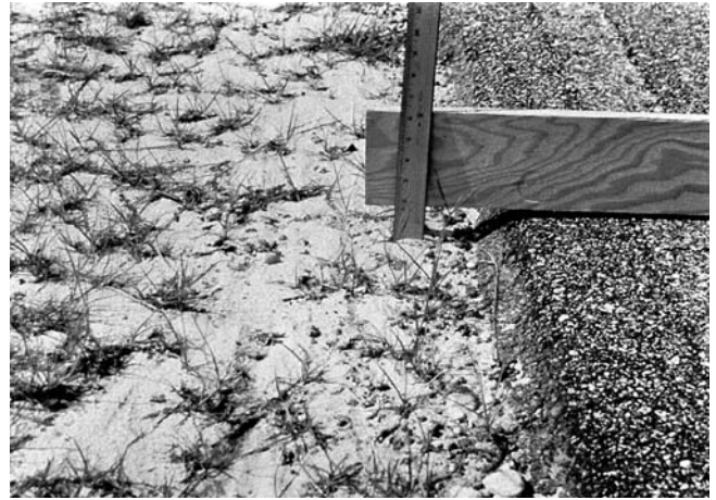
FIG. X1.25 Low-Severity Lane/Shoulder Drop-Off
