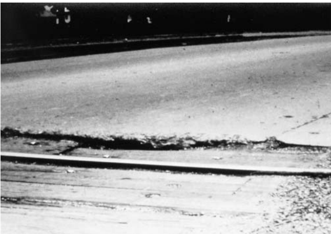
FIG. X2.40 High-Severity Railroad Crossing
