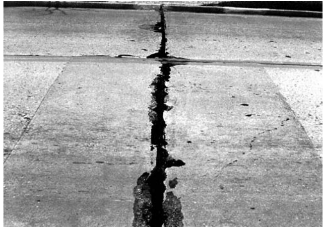
FIG. X2.16 Low-Severity Joint Seal Damage
