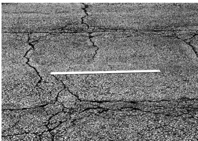
FIG. X1.7 Low-Severity Block Cracking
