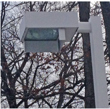
Figure 4. Even a modest shield can absorb a significant amount of the light from the luminaire and drastically reduce the luminaire efficiency.
