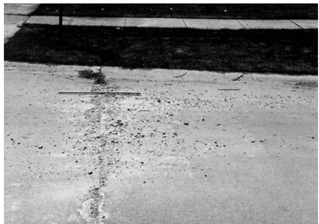
FIG. X2.1 Low Severity Blowup/Buckling
