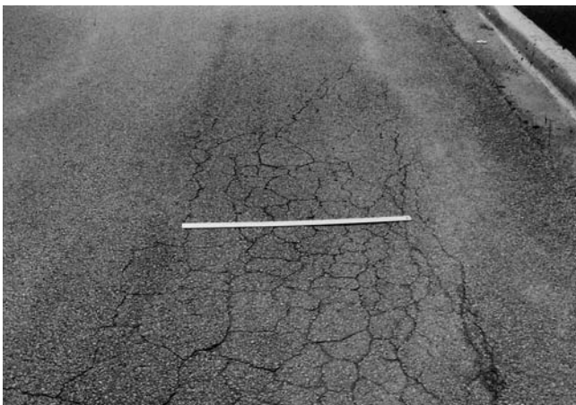
FIG. X1.2 Medium-Severity Alligator Cracking
