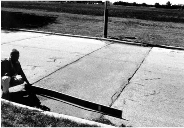
FIG. X1.32 Medium-Severity Patching and Utility Cut Patching
