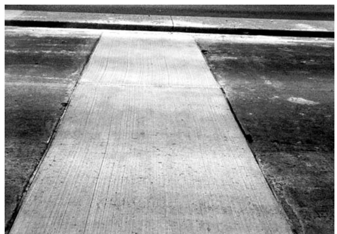
FIG. X2.25 Low-Severity Patching, Large and Utility Cuts
