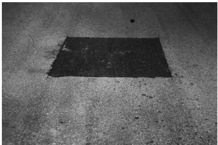
FIG. X1.31 Low-Severity Patching and Utility Cut Patching
