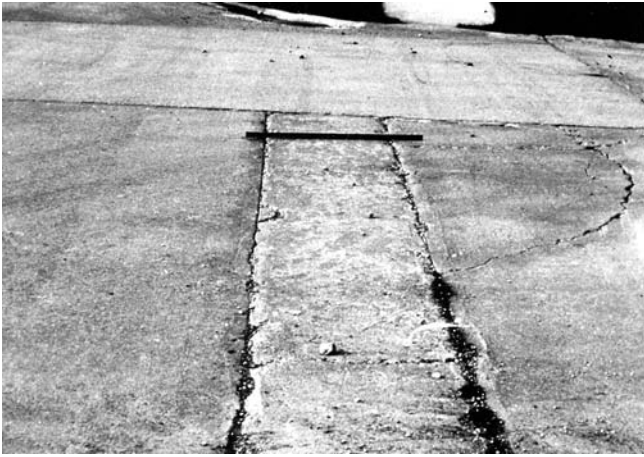
FIG. X2.26 Medium-Severity Patching, Large and Utility Cuts
