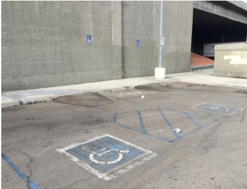
Photo 221: Non-Compliant ADA Ramps
