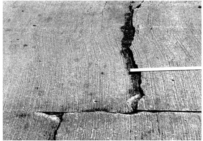
FIG. X2.24 High-Severity Linear Cracking
