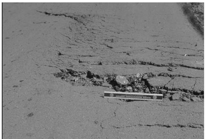
FIG. X1.49 High-Severity Slippage Cracking
