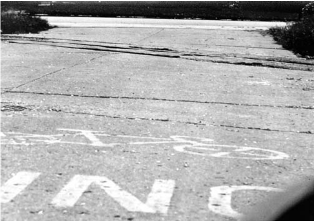
FIG. X2.39 Medium-Severity Railroad Crossing
