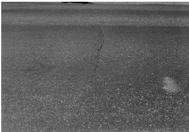
FIG. X1.28 Low-Severity Longitudinal and Transverse Cracking
