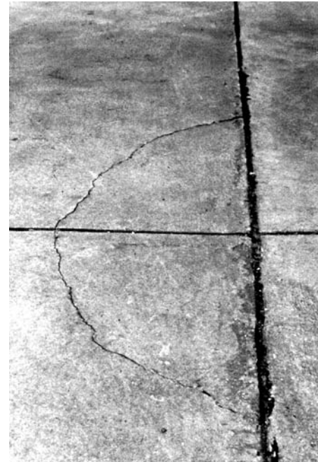
FIG. X2.4 Low-Severity Corner Break
