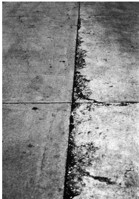
FIG. X2.49 Medium-Severity Spalling, Joint
