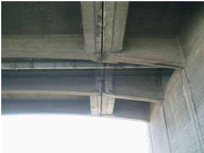
C. View of hinge crevices beneath the Willow Street Bridge over the Los Angeles River (06/23/09).
