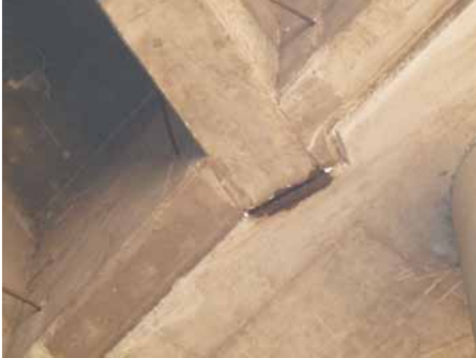
A. View of fresh staining at a small gap in an otherwise sealed crevice beneath the SR-91 bridge over the Los Angeles River (06/19/09).
