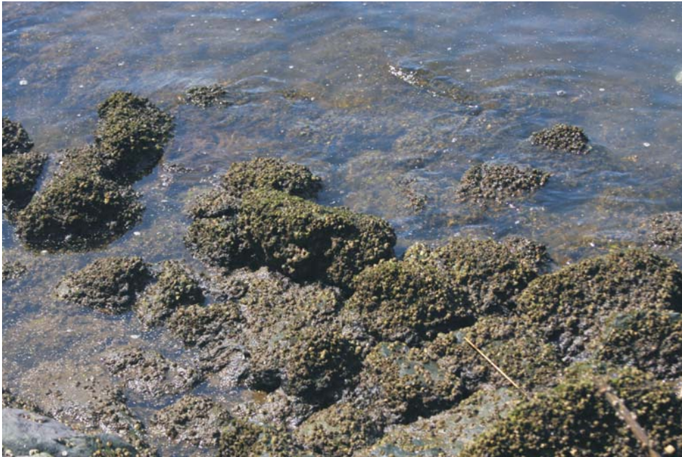
Figure 11 - Clusters of barnacles on a sediment-covered riprap apron lining the river estuary's shoreline.
