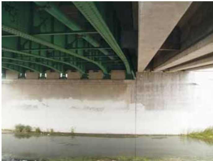
G. View beneath the Firestone Boulevard Bridge over the Los Angeles River, which consists of girders that may be used by night-roosting bats (06/15/09).
