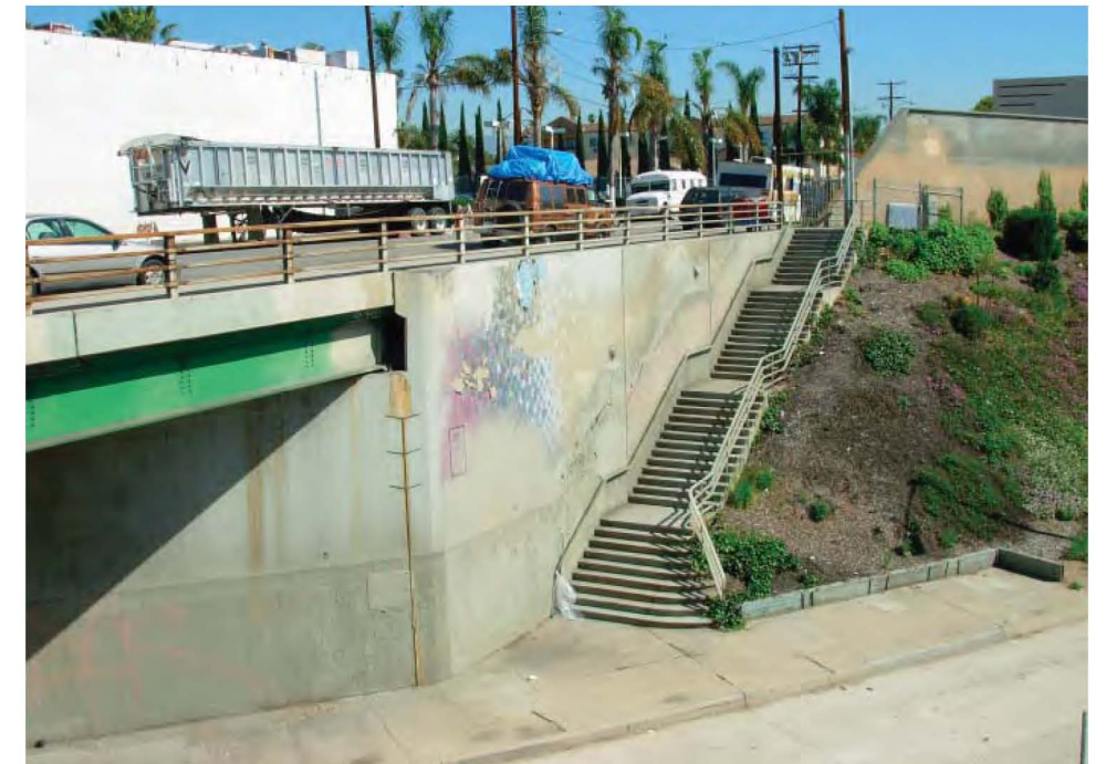
One of the many awkward edge conditions along the 101 freeway in Hollywood
