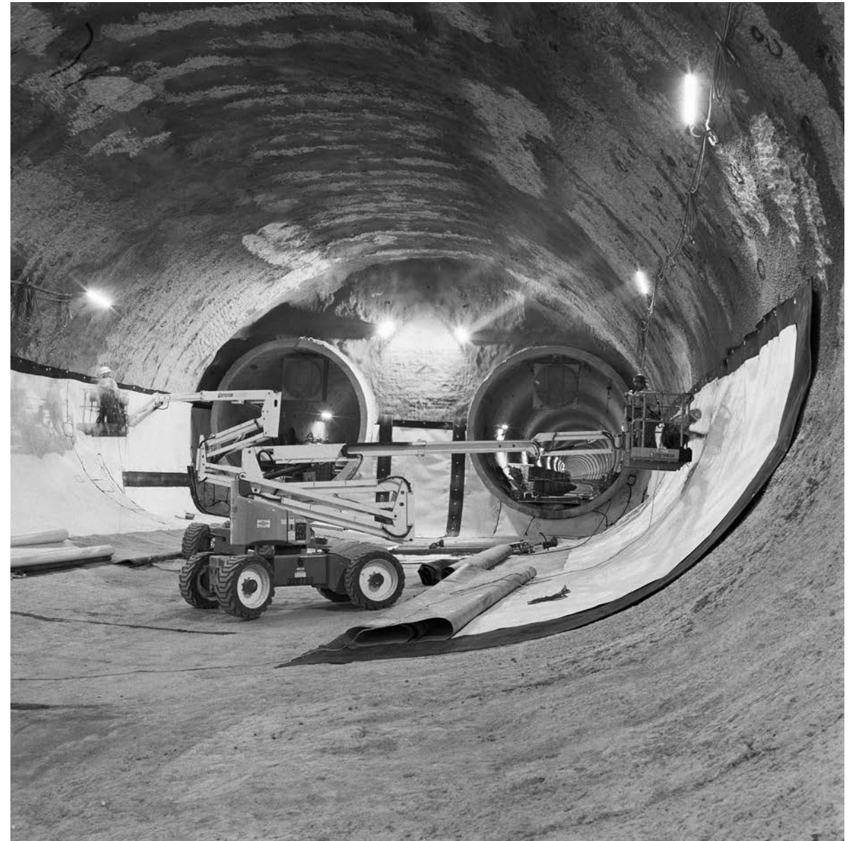
Workers install waterproof lining on the shotcrete lining surface of the Rail Crossover Cavern prior to the final lining installation.
