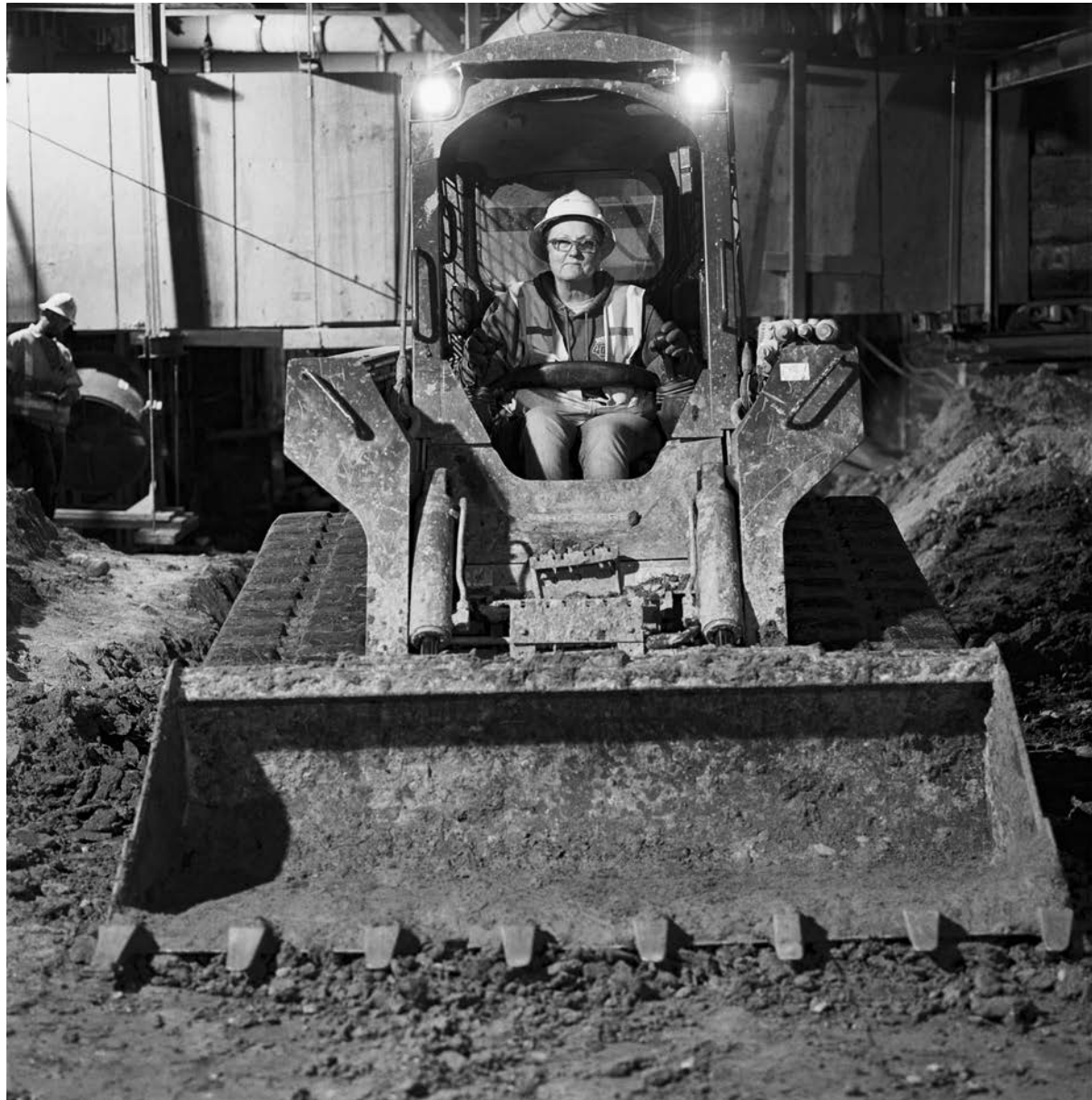
Lori Douglas, Heavy Equipment Operator, is removing the dirt for the “cut and cover” section of tunneling on the Regional Connector project.
