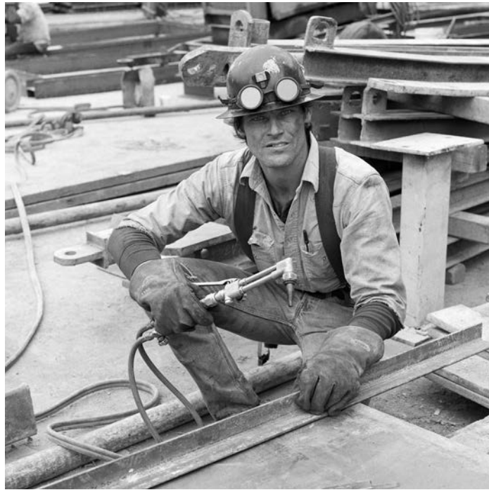
Pictured here at the Barnsdall topside construction site, Tony Anderson, a Tunnel Equipment Operator, worked many different tasks for the Red Line project from mining to welding, and as a mechanic.
