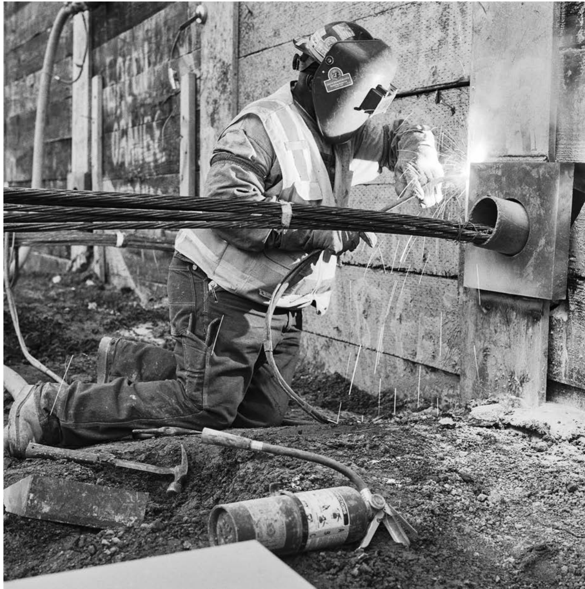
Karagozian relays, "A construction worker welding can make for a dramatic long exposure photograph. Here the worker is welding a tieback anchor collar to a soldier pile."
