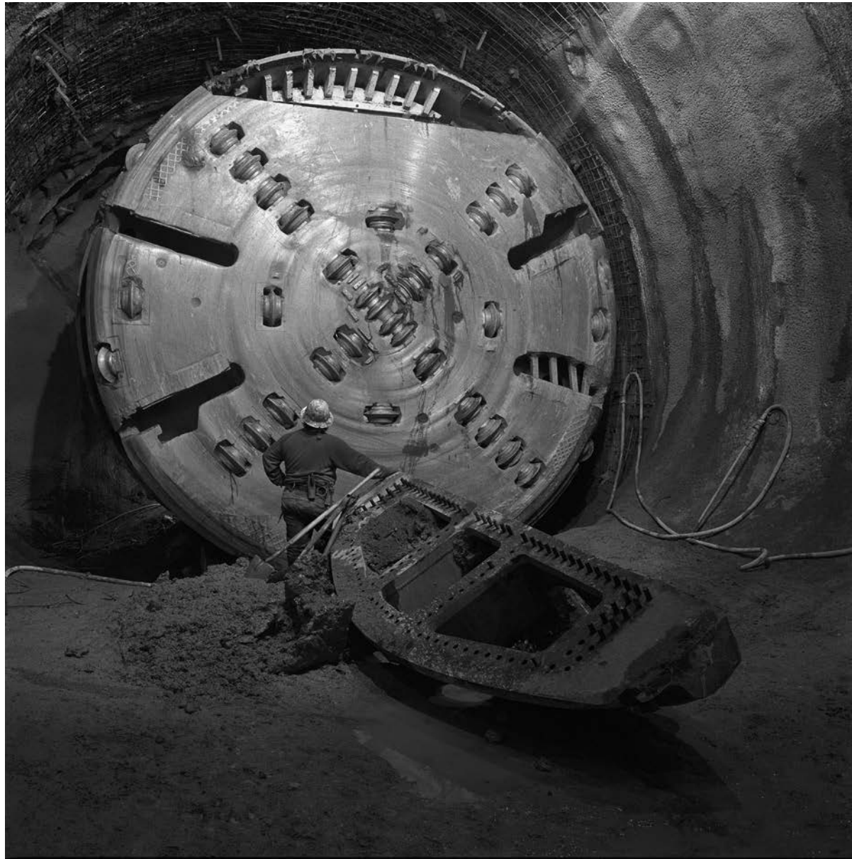
Thelma & Louise were the names given to the two mammoth TBMs that carved through 2.5 miles of rock beneath the Santa Monica Mountains to create the Red Line. Each machine was the length of a football field with a cutting diameter of 20.67 feet. The object in the foreground is one of the four outer sections of the cutterhead.
