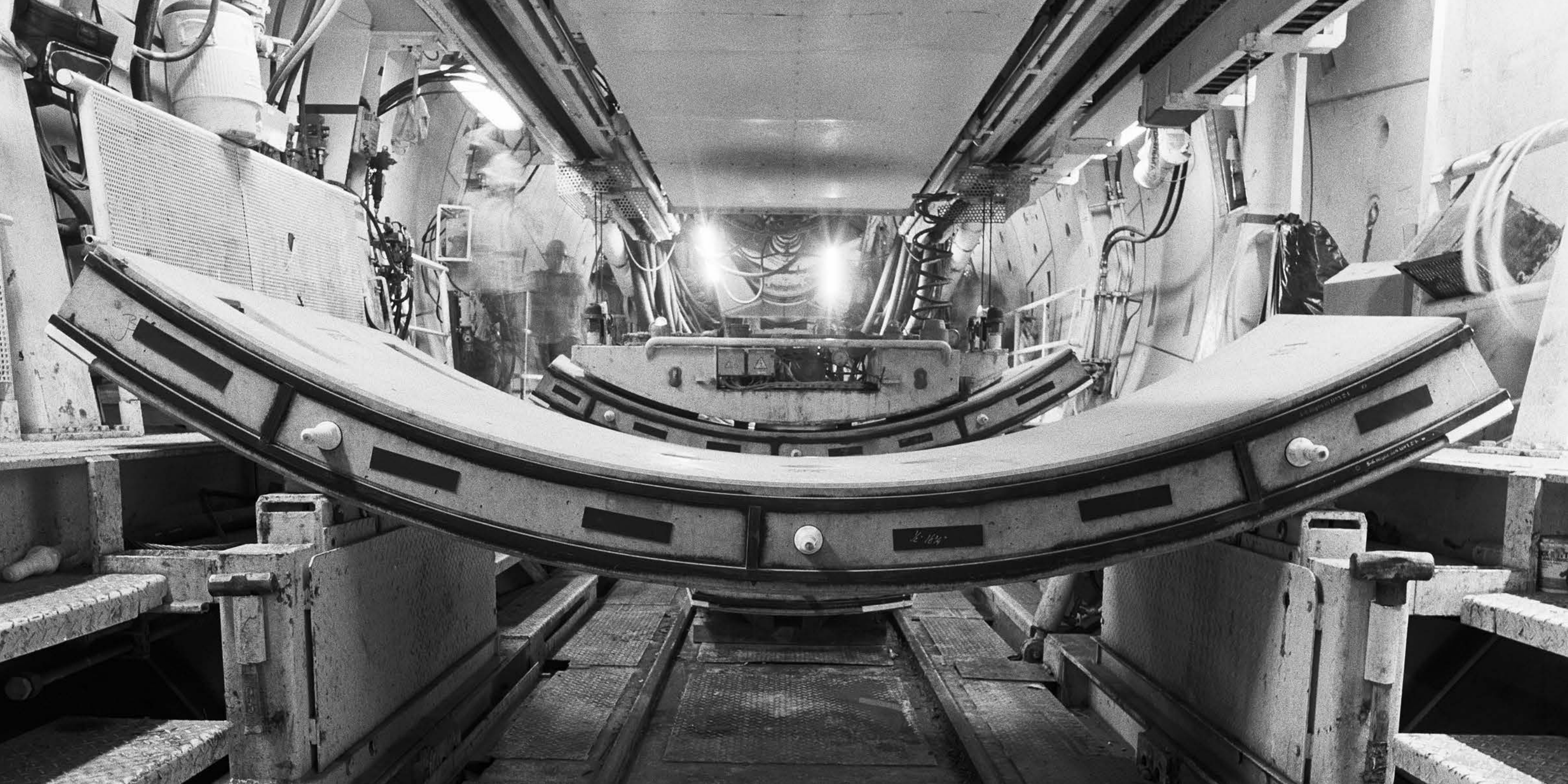
A view of the TBM tail with precast concrete tunnel lining segments that have double gasket joints to ensure a water and gas tight seal. The five-foot wide tunnel lining rings are assembled and placed as the TBM advances.
