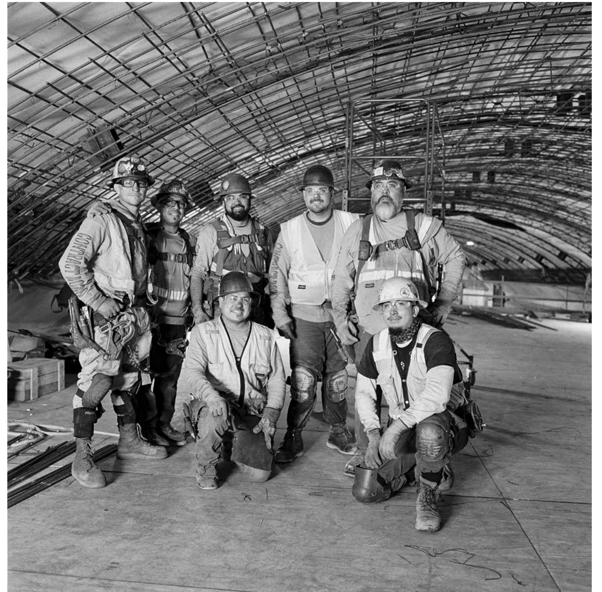
A group of ironworkers pose for a photo, after installing rebar on the crown of the cavern at the future station.
