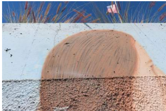
Photo 16: Hairline crack at southeast wall.
