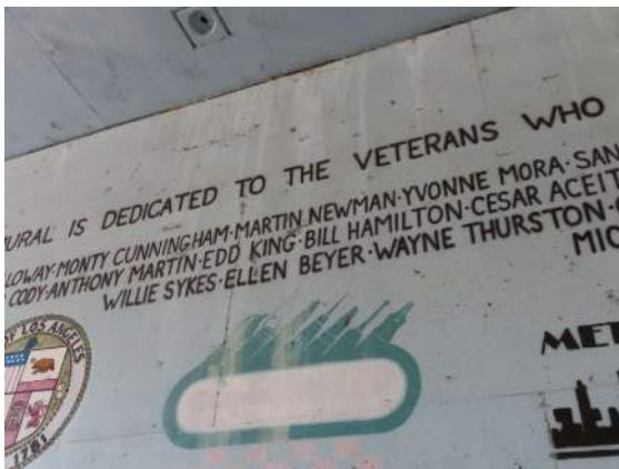
Photo 27: Detail of east elevation of Bonsall Ave. underpass; note drip stains and associated paint loss.
