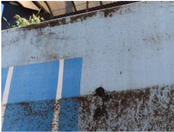
Photo 25: Detail at northwest wall; note heavy soiling.
