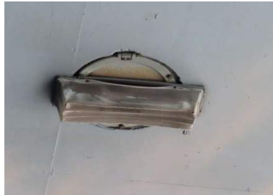
Photo 38: Light fixture at underpass ceiling.
