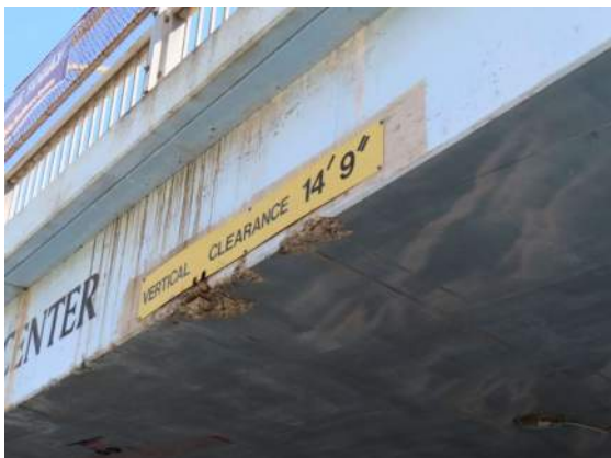
Photo 17: Detail of Bonsall Ave. underpass north entrance; note concrete spalling and corroded reinforcement, related to impact from trucks.
