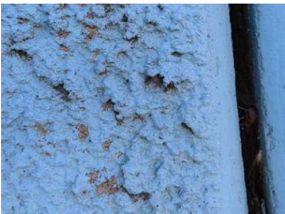
Photo 23: Detail at northeast wall; note paint loss, or possibly missing paint due to
