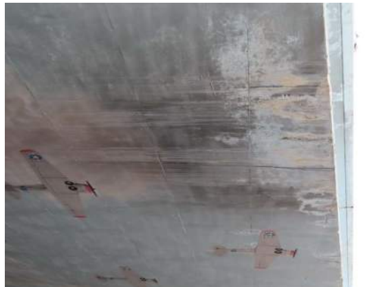
Photo 18: Detail of underpass ceiling at north entrance; note paint loss and abrasion damage from trucks.
