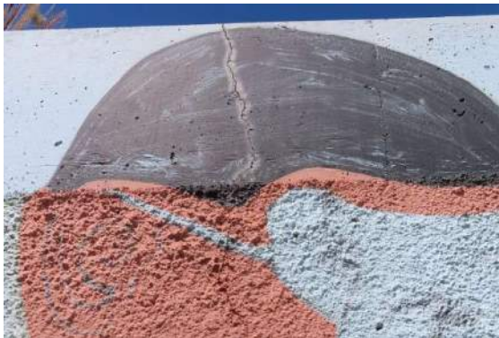
Photo 15: Crack at southeast wall, approx. 1/8-inch wide. Discoloration and paint loss at crack associated with water intrusion.
