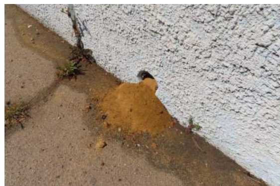
Photo 34: Detail at southeast wall; note soil erosion at drain hole.
