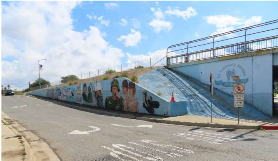
Figure 9 – Northeast retaining wall and corner slope (Wilshire Blvd. off-ramp, westbound). (source: ARG)
