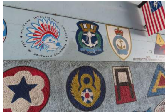
Photo 32: Detail at west elevation of Bonsall Ave. underpass; note overpaint, most likely to cover graffiti.
