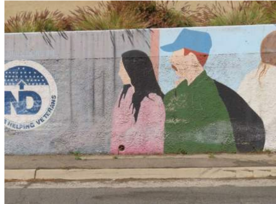
Photo 24: Detail at southeast wall; note paint loss at base of wall, possibly from prior
