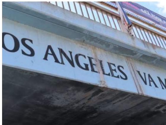
Photo 28: Detail of Bonsall Ave. underpass north entrance; note drip stains, efflorescence, and paint loss at bridge fascia and ceiling.
