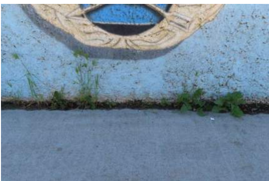
Photo 33: Detail at northwest wall; note plant growth.
