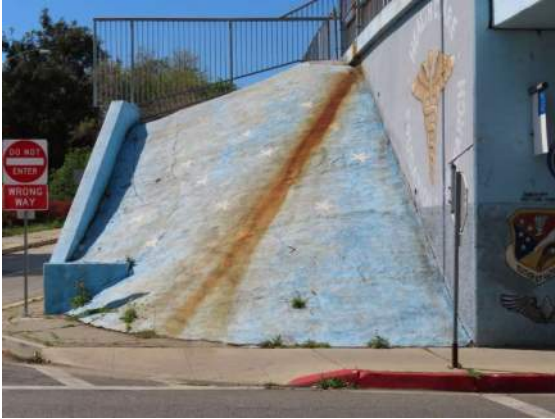
Photo 19: Southwest corner slope; note rust staining and eroded/faded paint.
