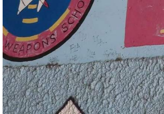
Photo 30: Detail of east elevation of Bonsall Ave. underpass; note writing/graffiti.
