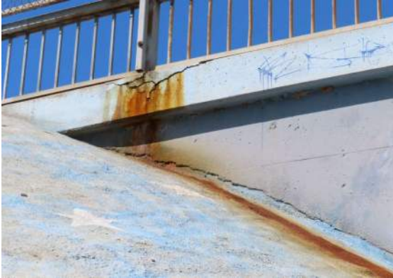
Photo 29: Detail at southwest corner slope; note rust stains associated with corrosion of embedded steel above.
