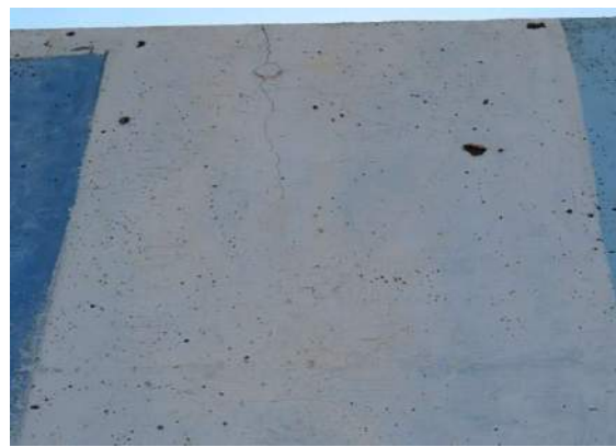
Photo 22: Detail at northeast wall; note cracking and peeling paint. Also note hairline crack above.
