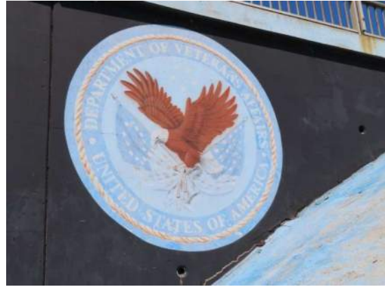
Photo 20: Detail of insignia at south elevation of bridge; note faded paint and lack of definition.
