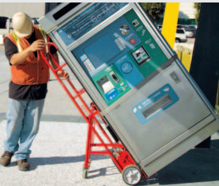
A worker rolls a ticket vending machine into place at the new Canoga station. The station extends the Metro Orange Line 0.3 miles.
