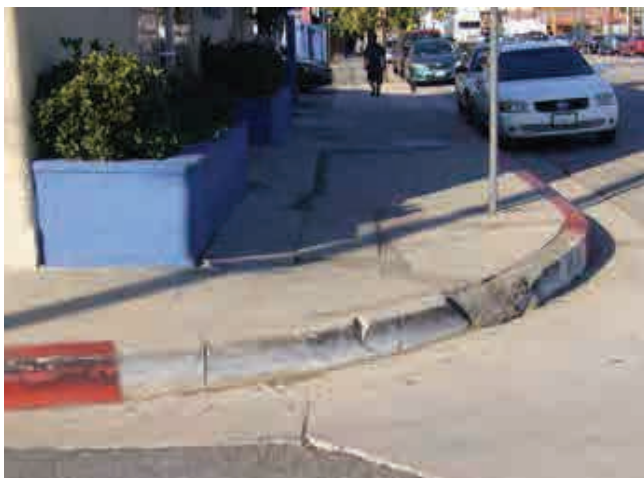
3.7 Lack of curb cuts
