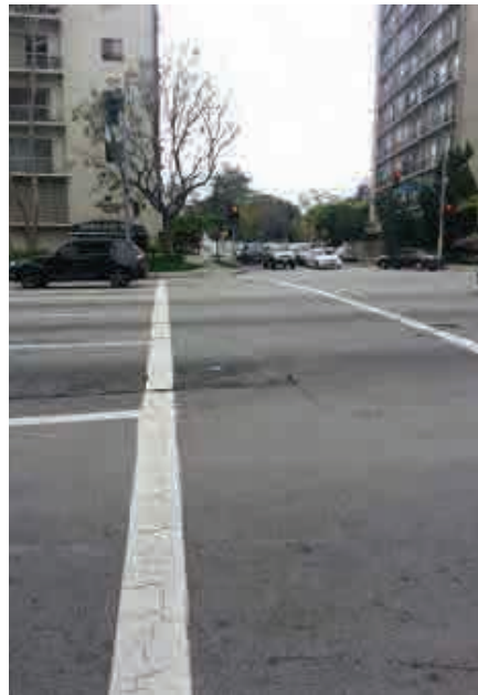
3.3 No pedestrian refuge at large crossings
