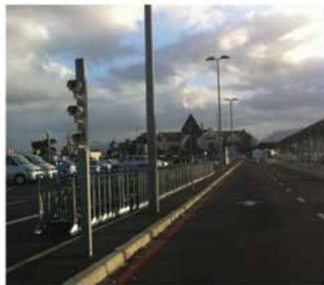
Lower end, single pole, side fire (South Africa)
