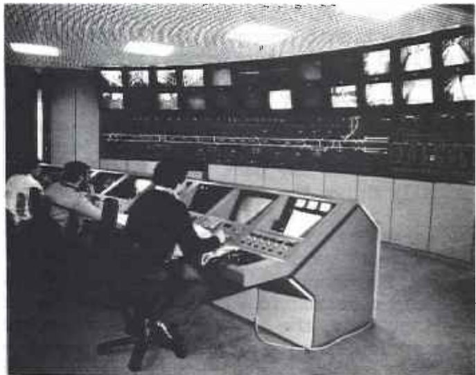
Central Control Center
