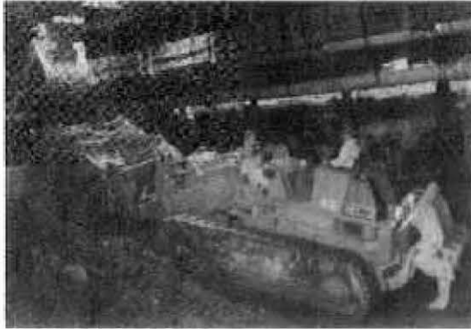
STATION EXCAVATION. CAT 977 LOADER, PILING MUCK TO BE LOADED OUT BY KOMATSU BACKHOE
