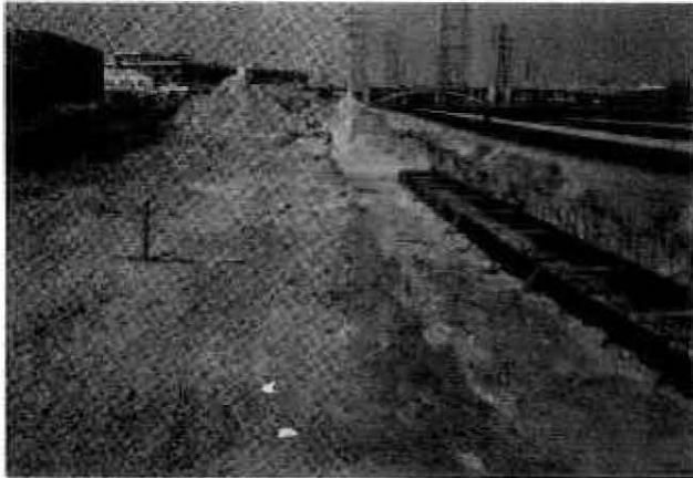
FORMING FOOTING FOR EAST RETAINING WALL, LOOKING NORTH TOWARDS MACY ST. BRIDGE
