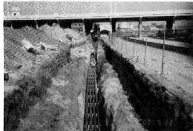
INSTALLATION OF TRACTION POWER DUCT BANK ALONG EAST R/W, SOUTH OF 1ST ST. BRIDGE
