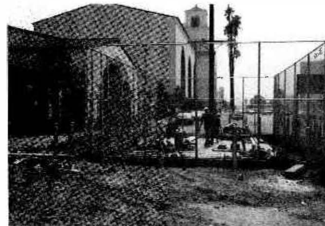
INSTALLING TRANSFORMER PAD AT UNION STATION TO PROVIDE POWER FOR TUNNELING AND DEWATERING OPERATIONS
