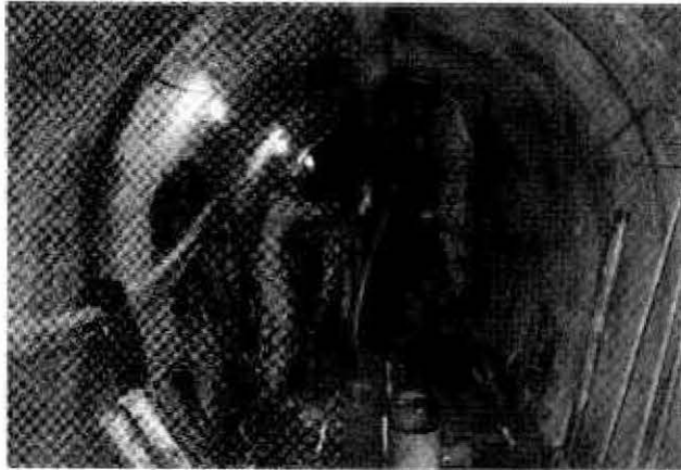
CORE DRILLING GROUT HOLES IN THE 9 FOOT DIAMETER STORM DRAIN AT THE INTERSECTION OF MACY AND ALAMEDA STREETS IN PREPARATION FOR CHEMICAL GROUTING
