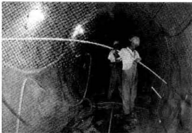
INSTALLING PVC CASING FOR CHEMICAL GROUTING IN STORM DRAIN AT MACY AND ALAMEDA STREETS
