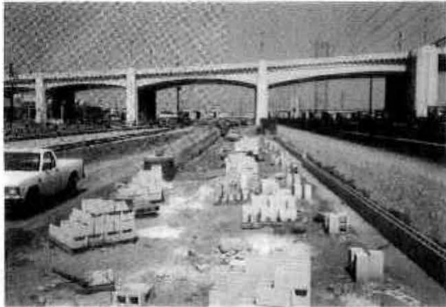
RETAINING WALLS AND LIGHT POLE FOUNDATIONS INSTALLATION, SOUTH OF 6TH ST. BRIDGE
