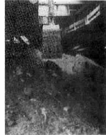
KOMATSU BACKHOE LOADING OUT MUCK FROM BELOW DECKING DURING STATION EXCAVATION OPERATIONS
