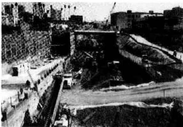
VIEW FROM ALVARADO ST. FACING EAST. SHOWS STATION EXCAVATION WEST OF WESTLAKE AVE. AND TEMPORARY HAUL RAMP
