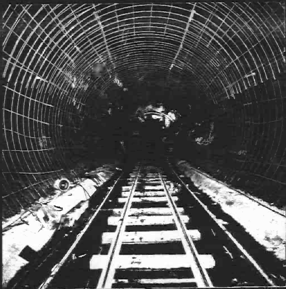
SLIDE A171-36 3/89 Arch reinforcement at A L tunnel prior to form and concreting. East view.
