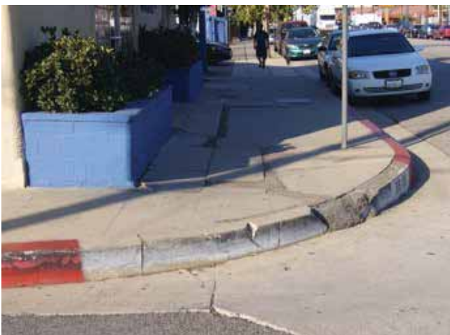
3.7 Lack of curb cuts
