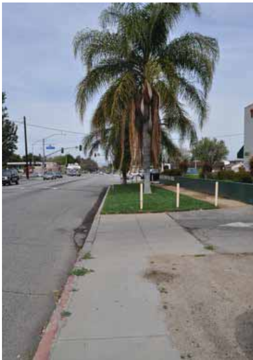
3.1 Discontinuous sidewalk along Newhall Ave. approaching Lyon Ave.
