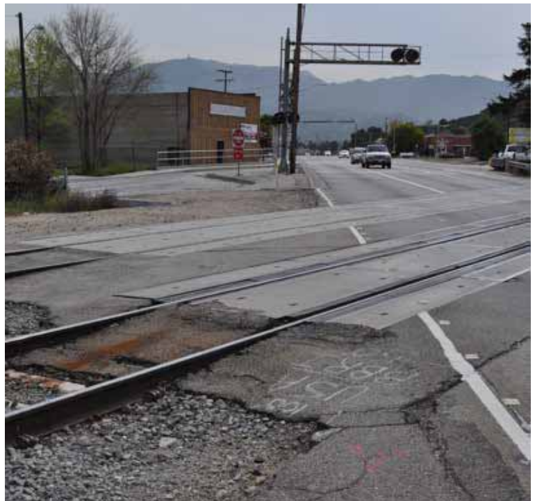
3.2 Non-accessible pedestrian path across tracks
